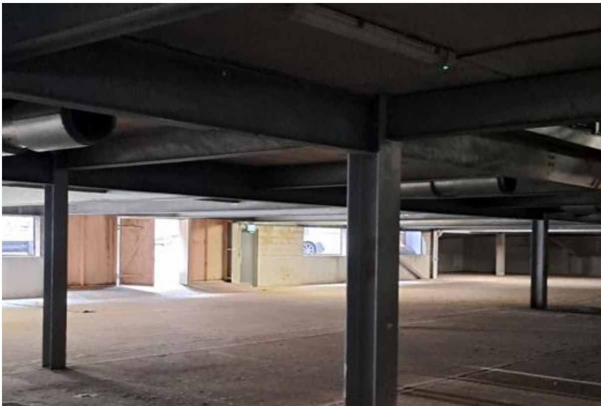
Figure 5. Lower ground floor of car park building light leak.
