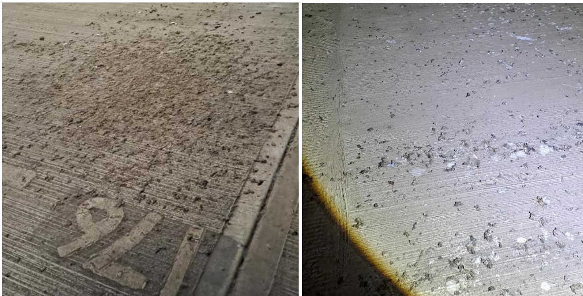
Figure 7. Evidence of previous bird presence on multiple levels.
