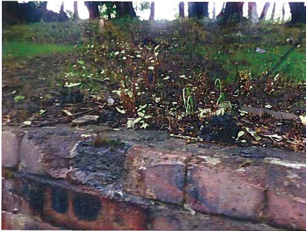
Dislodged Crown on site A
