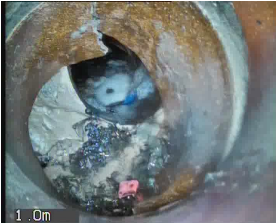
HOLX_40921092-5114-432d-b558-0fec6fb603fd_20230706_1 64509_567.jpg, 00:00:52, 1.20 m Collapsed drain or sewer, 75% cross-sectional area loss
