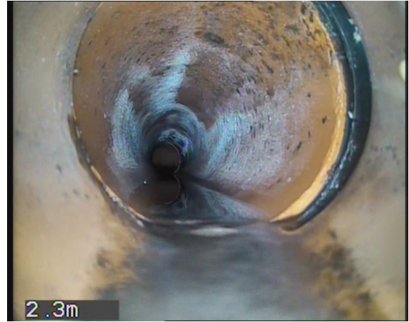
HOLX_ed093011-e2f5-4a5d-bb0a-c82d1728c269_20230706_152249_767.jpg, 00:00:29, 2.40 m Joint displaced, medium
