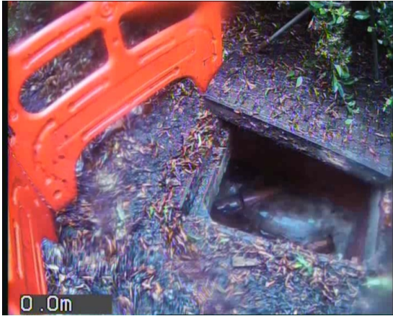
HOLX_8e91286a-d55b-4933-bf98-8effb2c1f404_20230706_1 63415_973.jpg, 00:00:00, 0.00 m Start node, manhole, reference: MH5 B1
