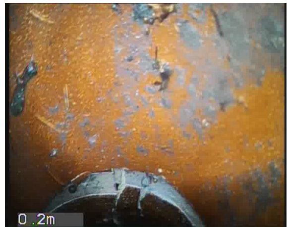
HOLX_76cc9b2a-b665-447d-95d1-72fa29e6e91d_20230706_1 64459_040.jpg, 00:00:38, 0.20 m Joint displaced, large
