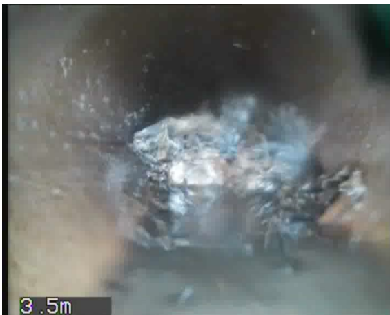
MH1X_d3511976-11b8-4d56-b062-5a1e811e0b99_20230706_150645_188.jpg, 00:00:46, 3.60 m Roots, mass, 75% cross-sectional area loss
