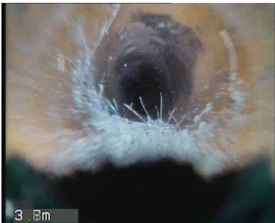
HOLX_e67ee152-1c09-4ec4-b448-c6d1fba0b59b_20230707_082517_066.jpg, 00:00:32, 3.90 m Settled deposits, fine, 10% cross-sectional area loss, Silt
