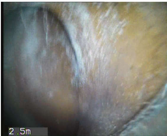
MH2X_077422f4-e6f4-4b0f-8667-8d31a5d6da3b_20230706_151144_037.jpg, 00:01:00, 2.50 m Line deviates down, Transporting drain
