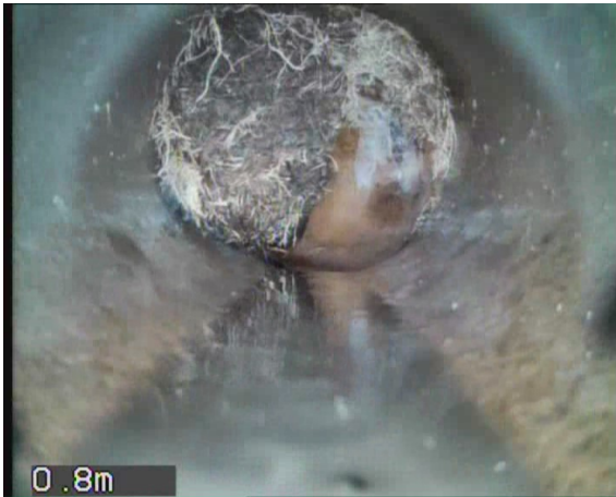
MH1X_aa273359-729b-4f23-940b-d8675b318ea2_20230706_150200_004.jpg, 00:00:18, 1.00 m Roots, mass at joint, 80% cross-sectional area loss
