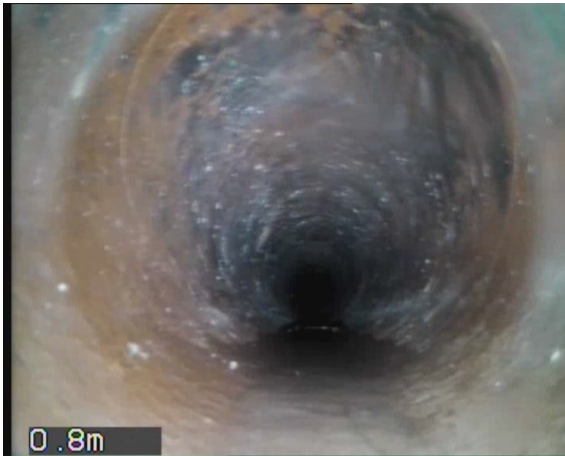
MH4X_cc020988-0011-4340-9d52-a30c5b3e12e1_20230706_161752_145.jpg, 00:00:24, 0.10 m Crack, circumferential from 8 o'clock to 4 o'clock
