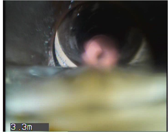
MH5X_487dd600-ffd7-4a9d-97c7-d70b5083bec7_20230706_162926_946.jpg, 00:00:27, 3.40 m Joint displaced, large
