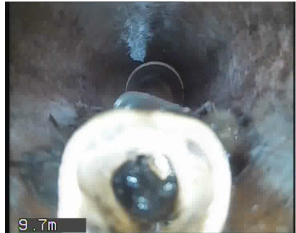
HOLX_bbddef19-5a48-4709-9377-e3b40a3892d7_20230706_141628_416.jpg, 00:01:45, 9.70 m Other obstacles from 5 o'clock to 7 o'clock, 20% cross-sectional area loss, Obstruction
