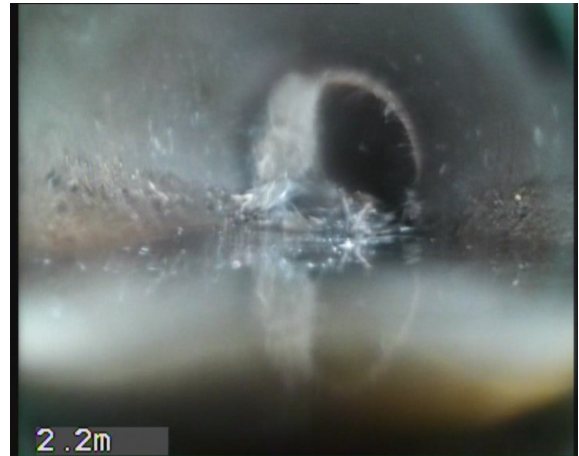
MH1X_4943f859-0f97-45a6-b8f1-ce69cc39453f_20230706_150613_957.jpg, 00:00:26, 2.30 m Water level, 40% of the vertical dimension
