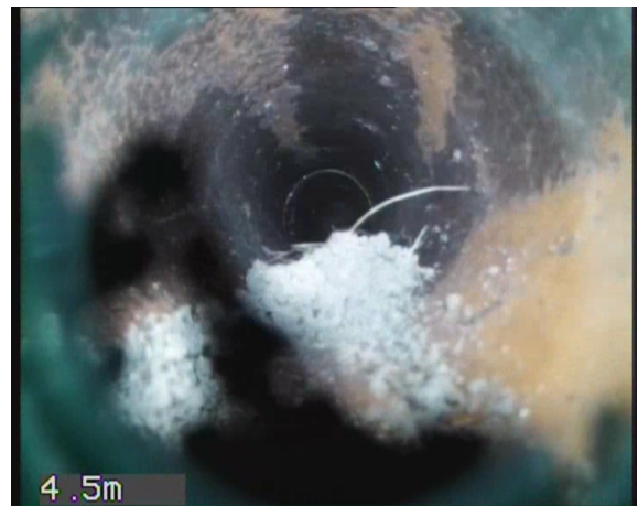
HOLX_89ff2a4d-168b-4738-b25e-0c54171b5712_20230707_082541_259.jpg, 00:00:40, 4.50 m Survey abandoned, Unable to pass silt
