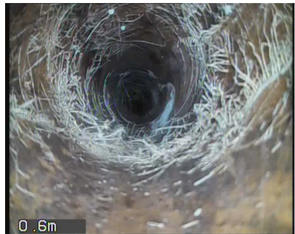
HOLX_b7094c9e-f71a-4390-8a2c-82a8b89ce3f7_20230706_144752_637.jpg, 00:00:39, 0.70 m Roots, fine at joint, to 1.8m
