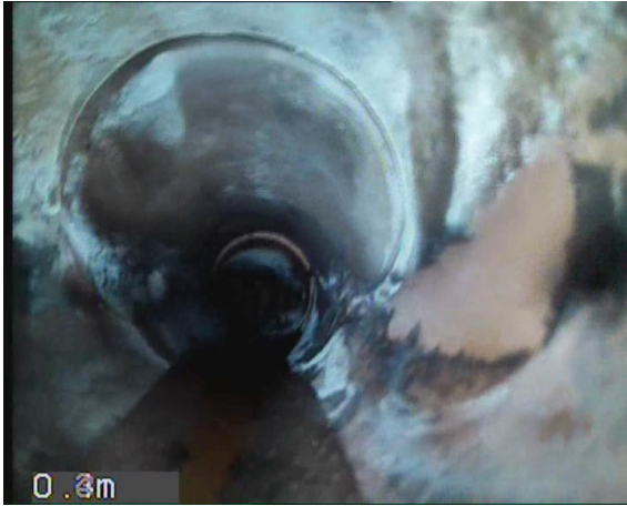
HOLX_3aa05ce1-21f2-4054-9a49-fd8b3a24f0d7_20230706_1 55614_563.jpg, 00:00:16, 0.40 m Crack, circumferential from 8 o'clock to 4 o'clock
