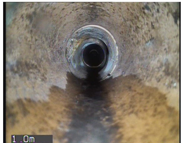
HOLX_fd025202-e33a-4a99-8644-b8ab0bc96fb6_20230706_141219_816.jpg, 00:00:38, 1.20 m Roots, fine at joint
