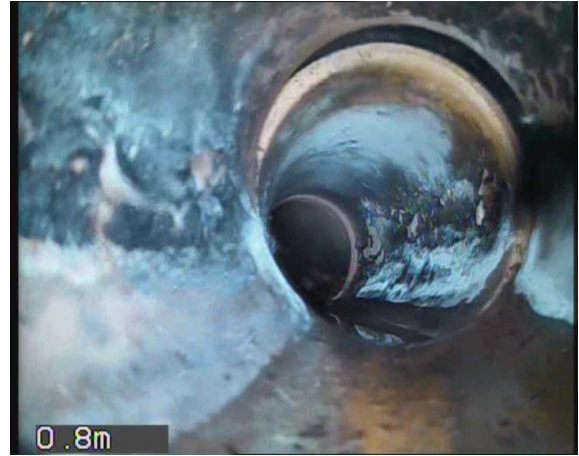
HOLX_24c842d0-7291-42a2-9a2d-4fe320ef24cf_20230706_1 55624_515.jpg, 00:00:19, 0.90 m Joint displaced, large
