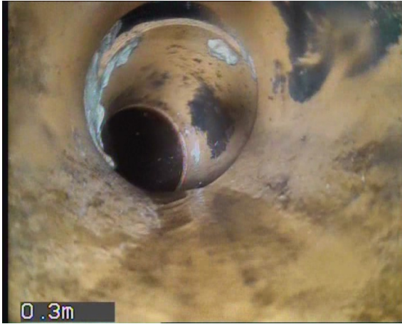
MH5X_fdccdda9-5e7a-4bf9-ad5b-b03a58808f1c_20230706_162759_472.jpg, 00:00:07, 0.50 m Joint displaced, large
