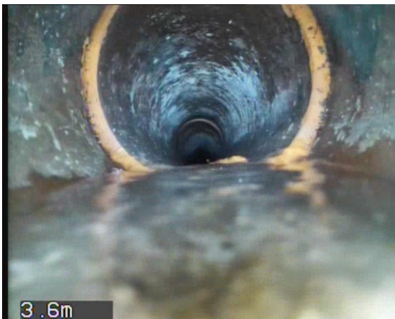
MH4X_18eae1b9-5507-4cfd-9d9e-79c916e211a7_20230706_162134_655.jpg, 00:00:49, 3.80 m Joint displaced, large
