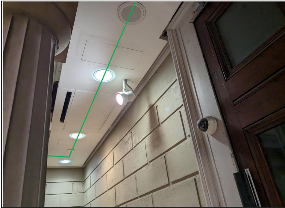
Appendix 13: The cable route continues toward GFAP3 using the false ceiling. As can be seen in the above photograph, several pieces of the false ceiling have been cut away for installation purposes and these may be utilized when running cabling through this historic area to minimize damage upon its character.
