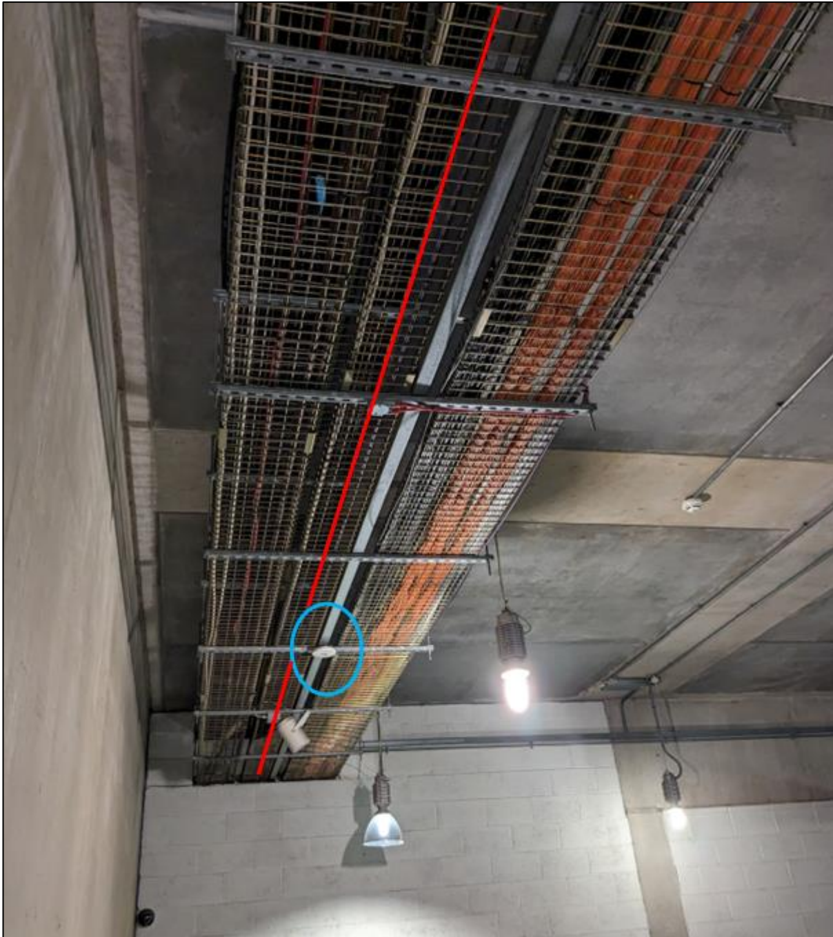
Appendix 25: GF021 Lading Bay, as pictured above, contains an existing steel conduit tray, along which existing network cabling runs (highlighted in red). An existing Wi-Fi access point, highlighted in blue, is to be replaced like for like with an up-to-date SDA model, GFAP10.
