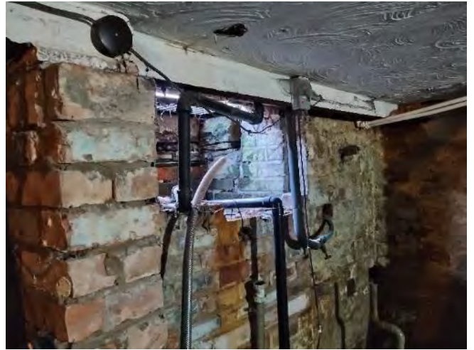
Figure 20 – Displays pipes leading from the sump onto the pavement level.
