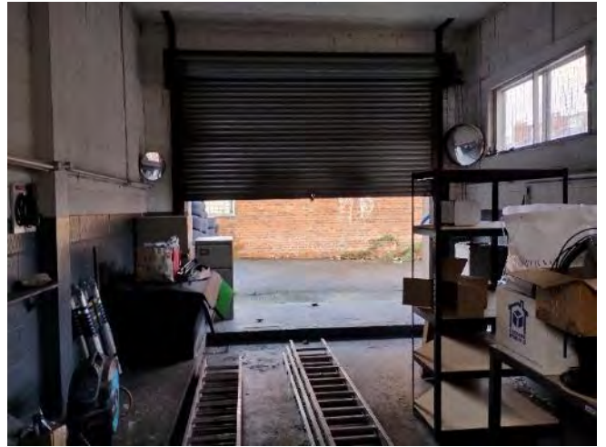
Figure 8 – Displays the garage section in the centre of the site. The centre of the floor is sunken 12cm below the rest of the garage level.
