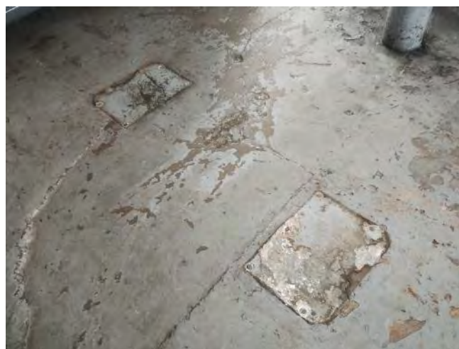
Figure 26 – Displays scarring in the concrete in the southern site section.
