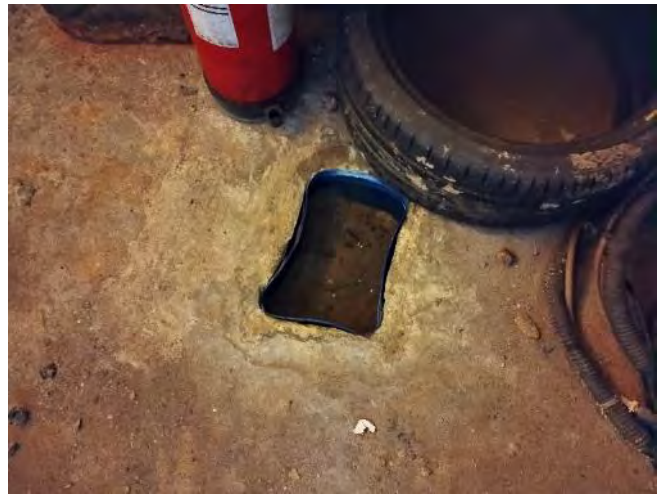
Figure 22 – A possible makeshift drainage solution within the basement.
