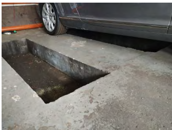
Figure 29 – Two sunken pits 30cm deep in the garage section
