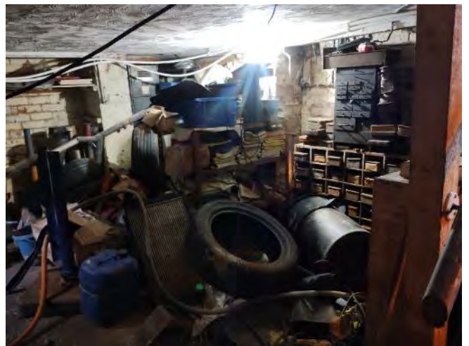
Figure 12 – A section of the basement displaying waste of tyres, metal and plastic drums, papers and boots.
