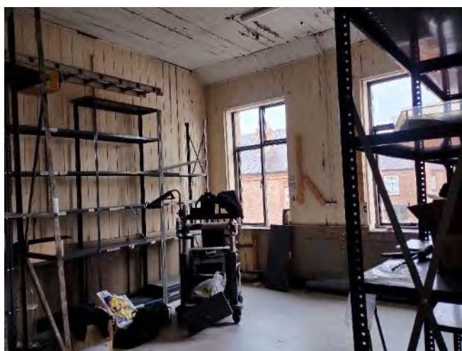
Figure 29 –The first floor of the garage showing the poor condition of the paint on the walls and ceilings.
