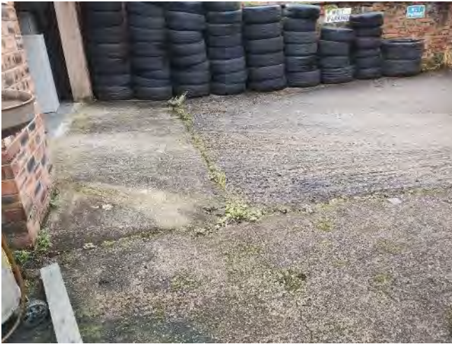
Figure 7 – Scarring in the hardstanding in the yard area.
