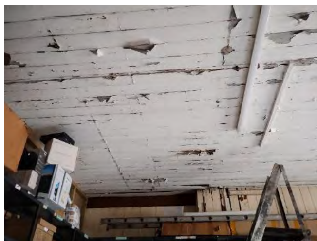
Figure 30 – Displays the flaking paint on the ceiling of the first floor in the southern section of the garage.
