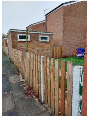
Photograph 21: Smashed garage windows along Lilstock Walk, south of the site.
