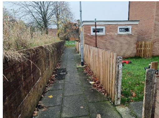
Photograph 22: Smashed garage windows further down Lilstock Walk, south of the site.
