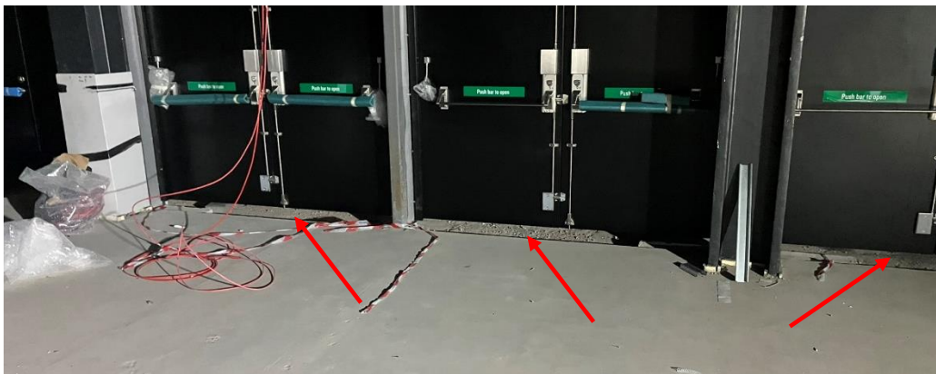
Figure 4 Gap under Atrium entrance doors (level M0)
