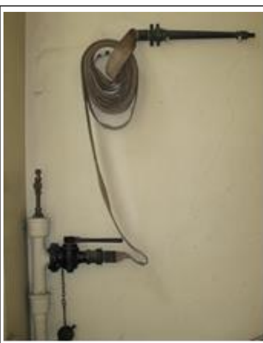
Example of 19 th Century Staircase Water Pipes and Firehose (Calke Abbey)
