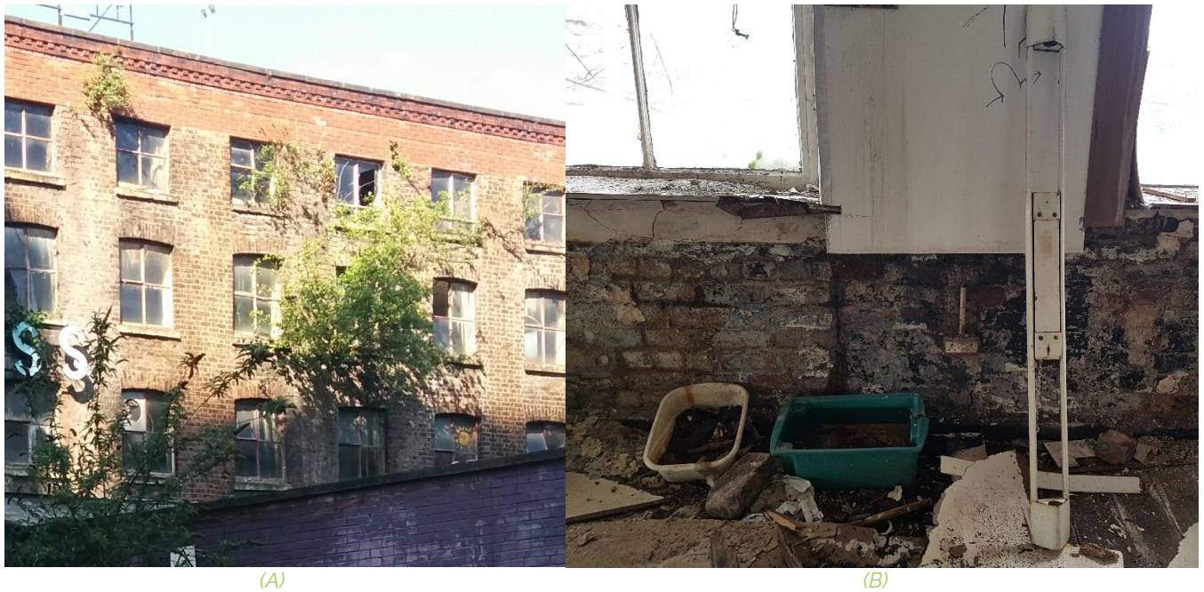
Figure 3 - Severe vegetation growth on eastern elevation (taken 2018)
