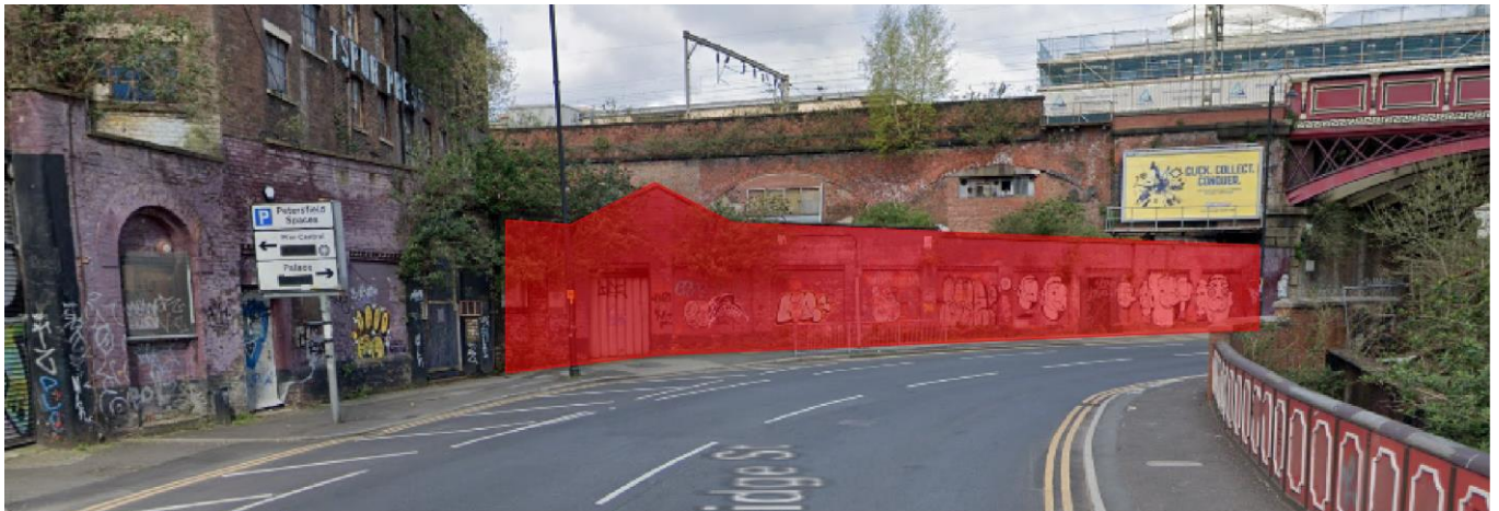
Figure 17 - Leaning wall + site access provision
