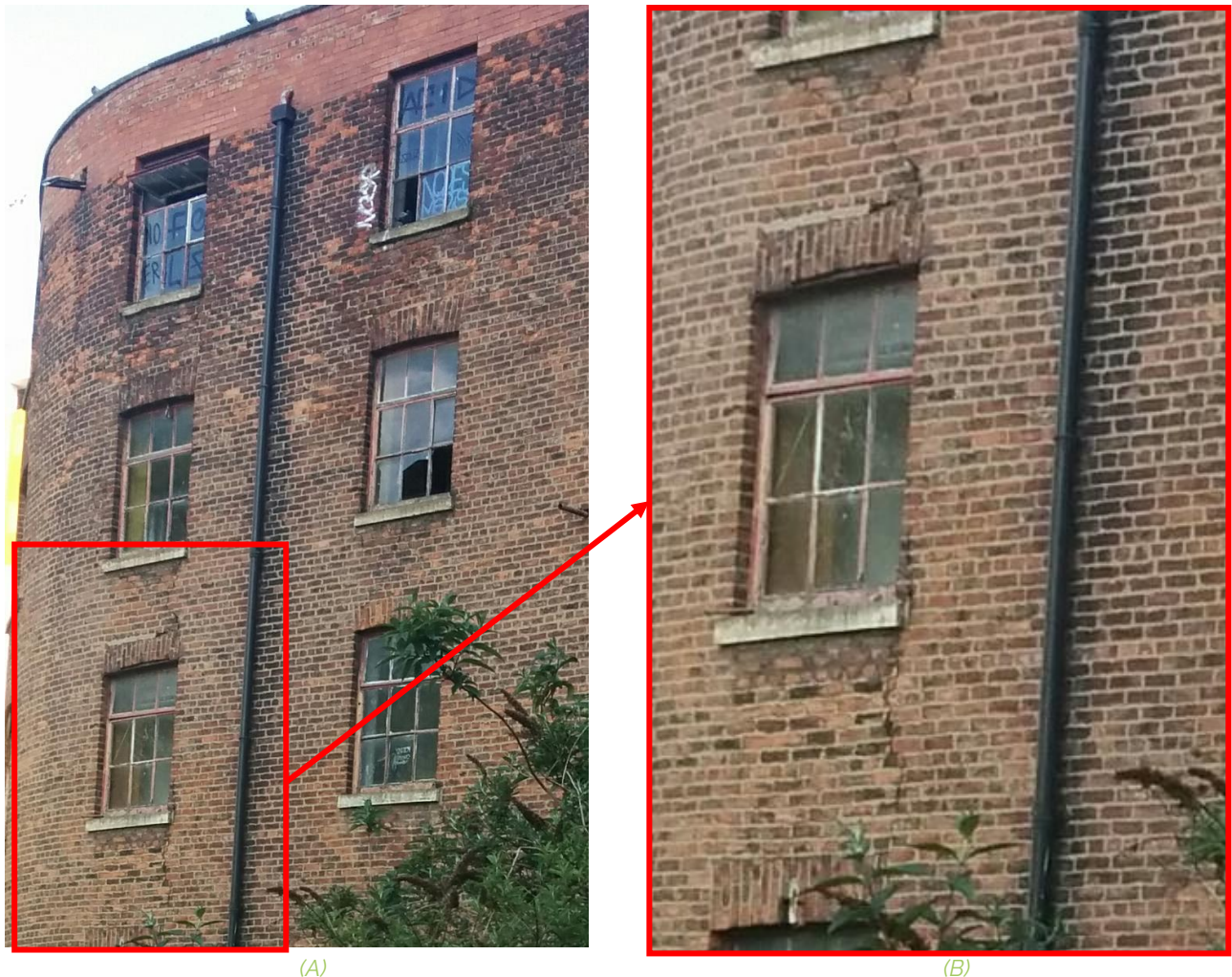
Figure 5 - Significant cracking on southern elevation (taken 2018)
