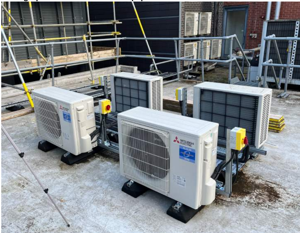
Photograph 1: Installed external equipment
