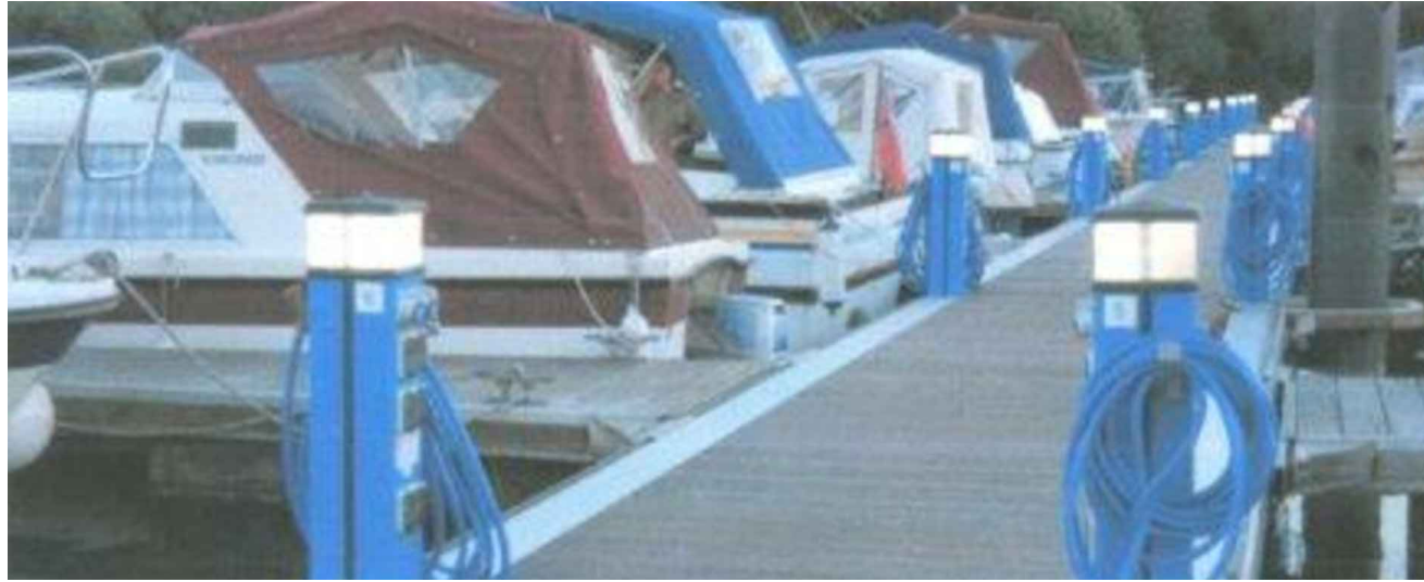
IMAGERY OF SERVICE PILLAR (ONE PER BOAT MOORING)
