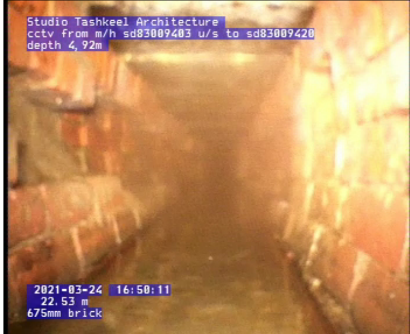
Photo: 1_1_20_A.jpg 22.53m, Missing bricks, from 7 to 5 o'clock, Start
