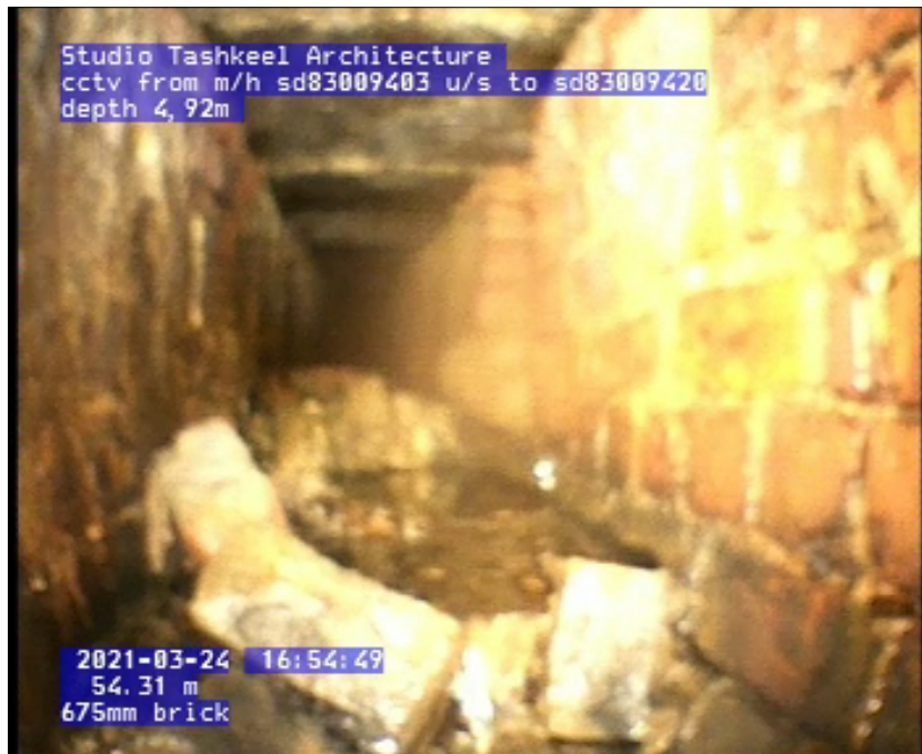
Photo: 1_1_47_A.jpg 54.31m, Settled deposits, coarse, 30% cross-sectional area loss
