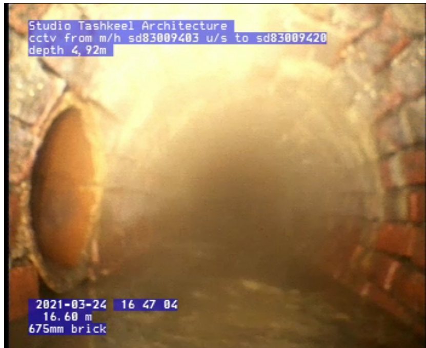
Photo: 1_1_14_A.jpg 16.6m, Connection other than junction, at 9 o'clock, diameter 225mm
