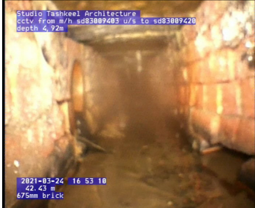
Photo: 1_1_34_A.jpg 42.43m, Missing bricks, at 5 o'clock
