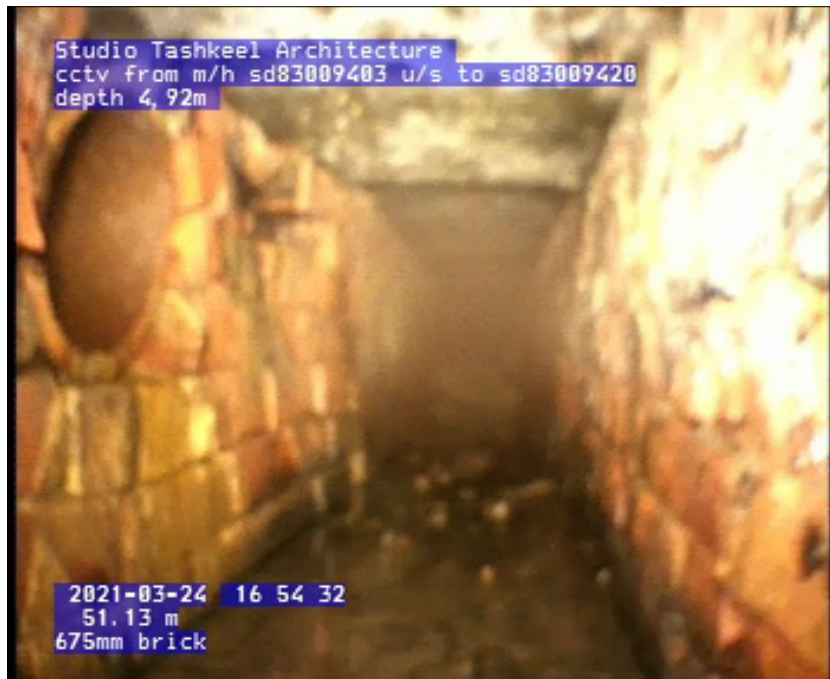
Photo: 1_1_40_A.jpg 51.13m, Connection other than junction, at 10 o'clock, diameter 150mm
