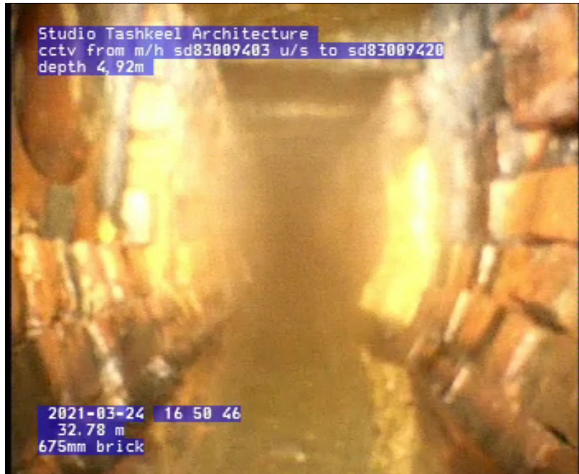
Photo: 1_1_25_A.jpg 32.73m, Connection other than junction, at 10 o'clock, diameter 150mm
