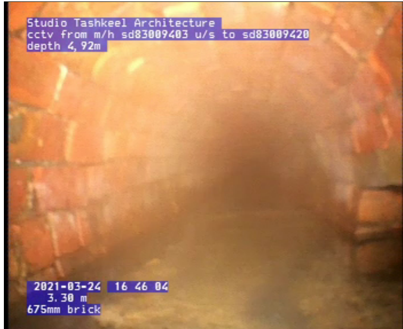
Photo: 1_1_8_A.jpg 3.3m, Missing bricks, from 3 to 4 o'clock
