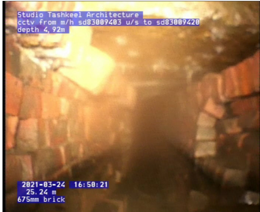
Photo: 1_1_22_A.jpg 25.21m, Displaced bricks, at 11 o'clock
