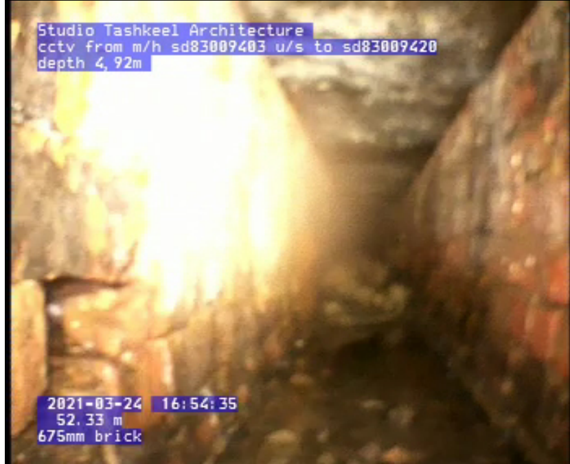
Photo: 1_1_41_A.jpg 52.33m, Missing bricks, at 9 o'clock
