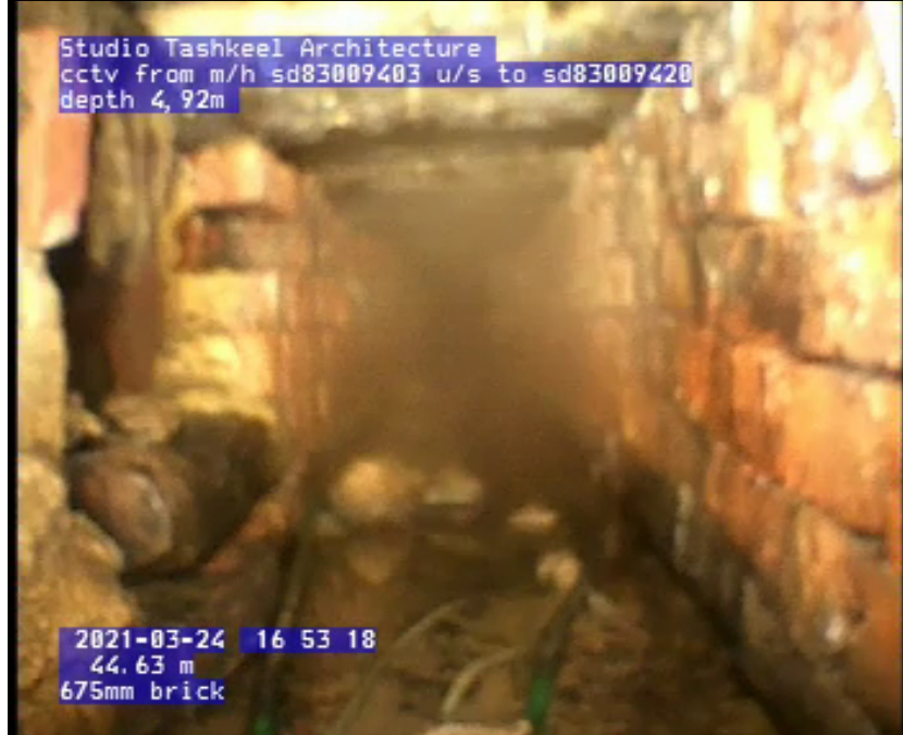
Photo: 1_1_36_A.jpg 44.63m, Missing bricks, from 7 to 11 o'clock
