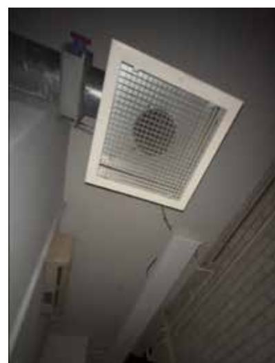
Figure 4.4 Basement: existing fresh air services to ceiling.
