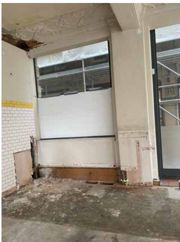
Figure 4.21 Ground floor: modern wall tiles to be removed from modern plasterwork. Area of damage on wall to be made safe and painted only.
