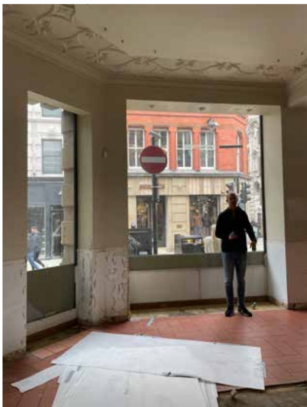
Figure 4.15 Ground floor: all columns have modern plaster attached and to be made good.
