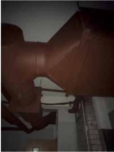
Figure 4.5 Basement: existing services to ceiling.
