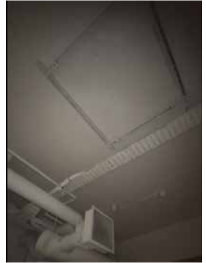
Figure 4.7 Basement: existing fresh air service to ceiling in northern room (along Cross Street).
