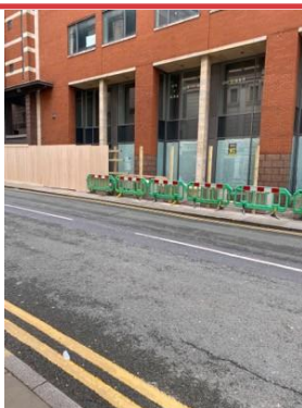
ISSUE 1 Highway photograph showing existing cracking to tarmac and hoarding being constructed on footpath - Quay Street looking towards Deansgate A56
