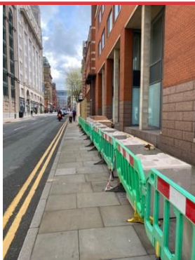
ISSUE 3 Footpath photograph showing minor displacement of paving slabs, hoarding being constructed on footpath and temporary barriers installed - Quay Street looking towards Deansgate A56
