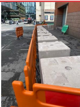
ISSUE 4 Photograph showing existing cracking and patching to carparking bays and footpath. Concrete blocks and temporary barriers placed in preparation for hoarding erection – Byrom street looking towards Quay Street.
