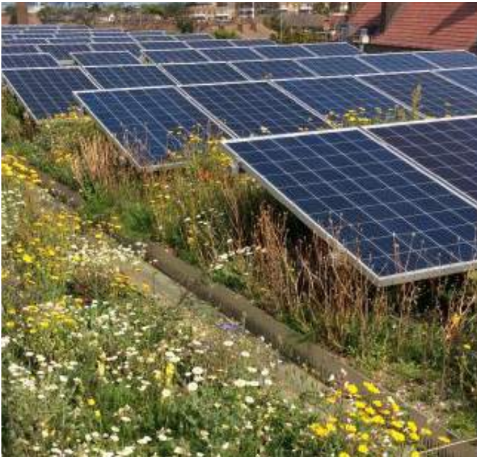
Biosolar roof system
