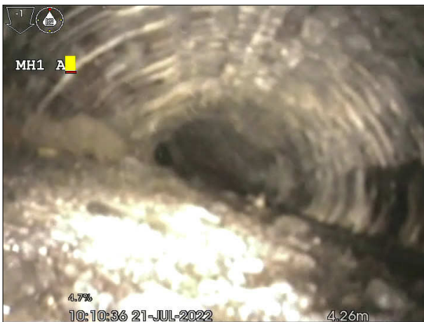
Photo: 1_6a, 00:00:00 4.26m, Debris silt, 35 % cross-sectional area loss, Changed
