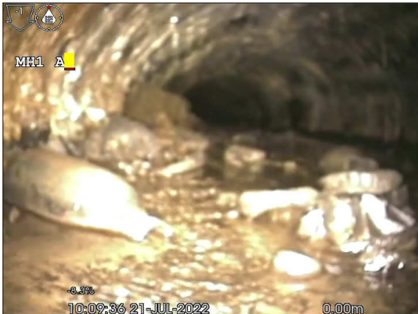
Photo: 4_4a, 00:00:00 0.2m, Debris silt, 25 % cross-sectional area loss, Start
