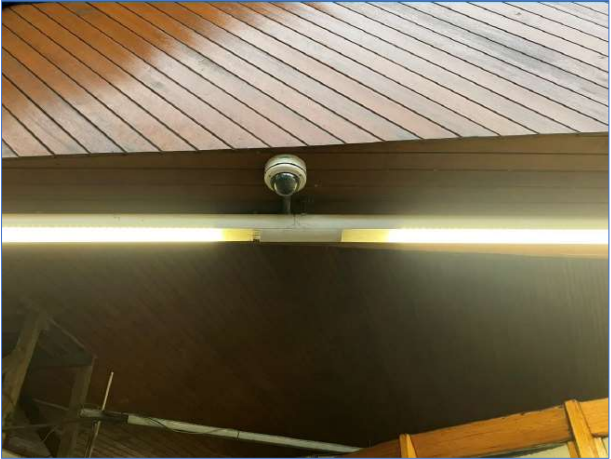
Figure 11 - Existing dome camera with conduit hidden from view behind existing strip lighting
