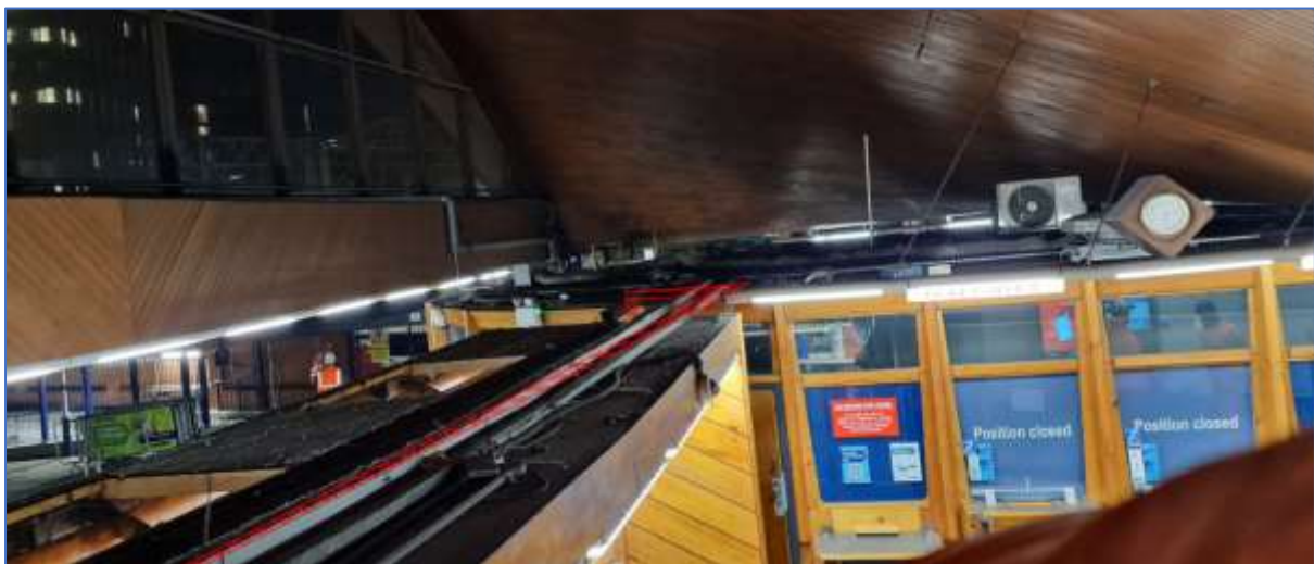
Figure 4 - Cable route above station entrance doors (security room at bottom of image, behind camera)
