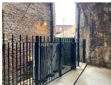
Image 4: Access to arch/ ASHP's
