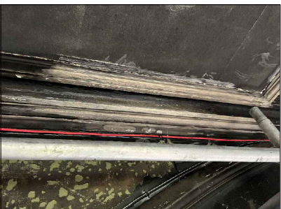
3&4 coving colours have been lost (replicated from photos)
