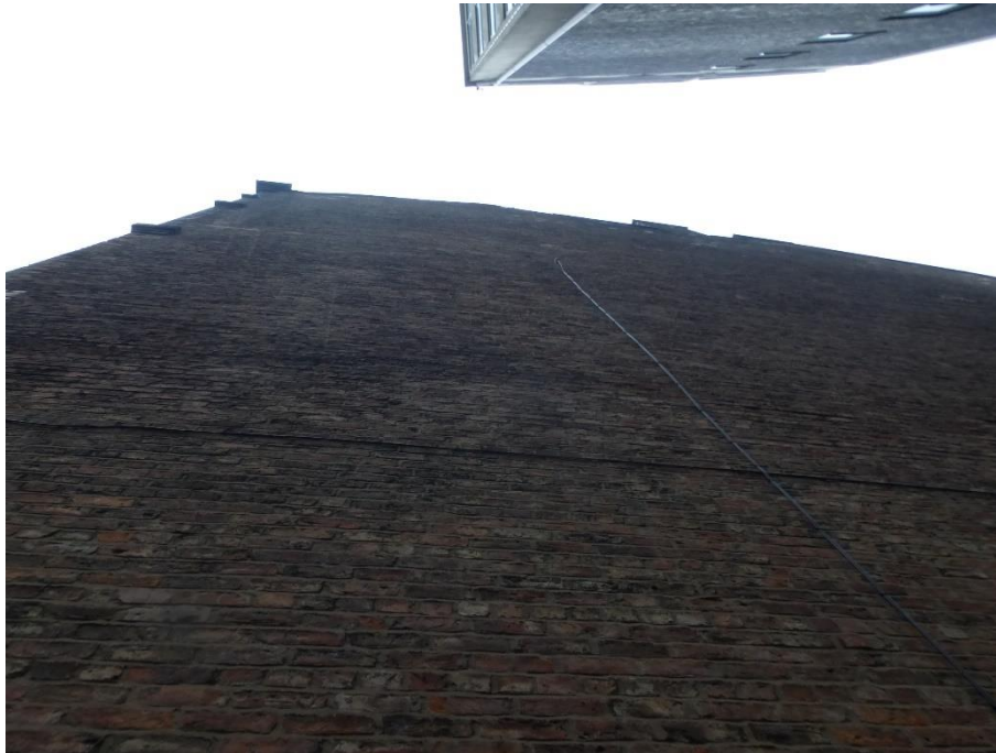
Small areas of misalignment can be seen on the gable wall, but not excessive
