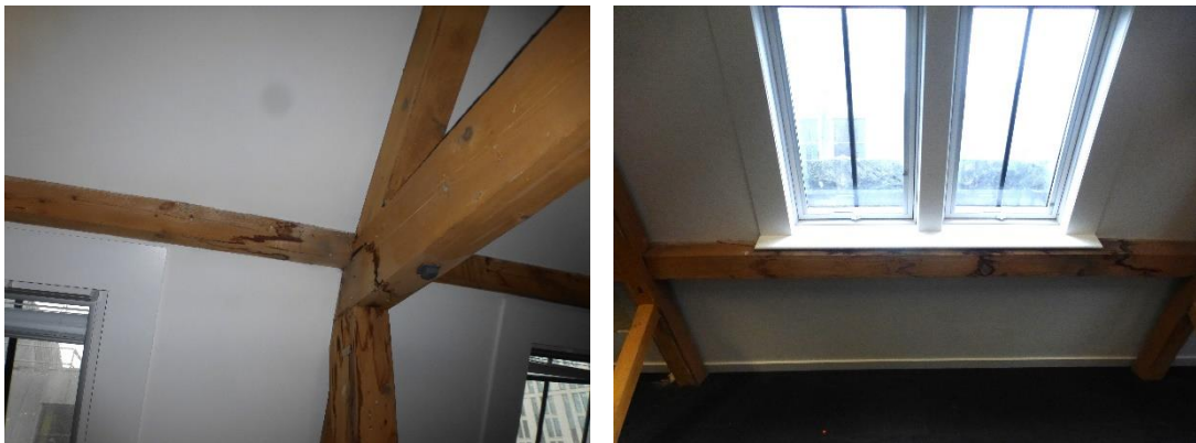
Water staining to timber trusses and purlins at 4 th floor level.
