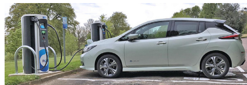
Indicative Electric Vehicle Charging Bay
