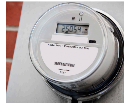
Indicative Smart Electric Meter
