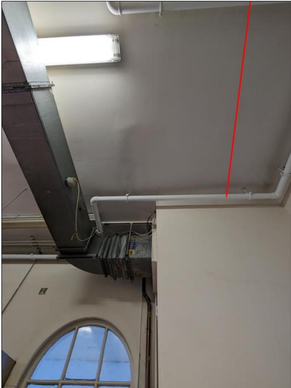
Appendix 14: As mentioned in Appendix 13, the cable run passes via the loft space between 002 Circ. and 016 Kitchen. Photographed above, the cable enters 016 Kitchen via 002 Circ. and using the ceiling void is routed through the wall facing the Café area (as seen in Appendix 15).
