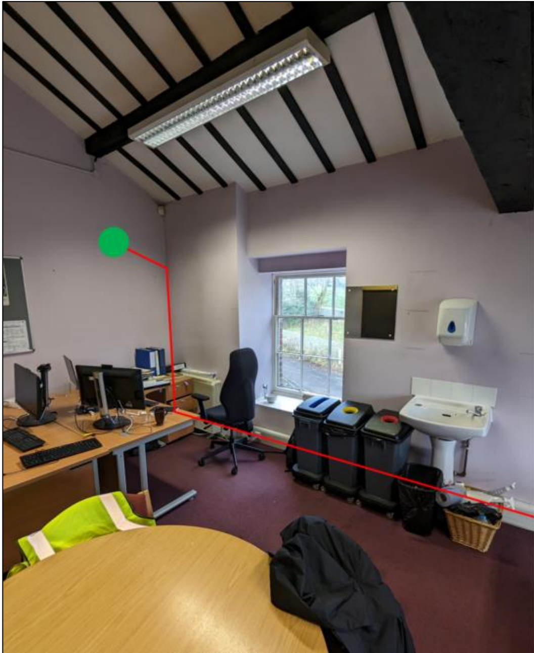
Appendix 7: The photograph above, taken in 014 Office, illustrates the continuation of the cable run detailed in Appendix 6 with its termination at the point marked by a green circle indicating the point at which an access point is to be installed. The cable run primarily utilizes an existing stretch of trunking and will then use a steel conduit to run up the wall and provide network connection to the access point.
