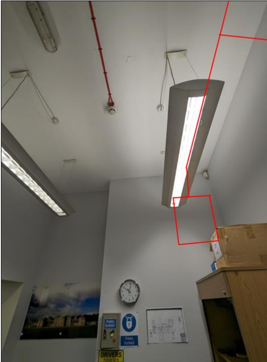
Appendix 9: GF030 Office, pictured above, shows a second cable running from the point at which the run enters the loft void, as opposed to the first which terminates with AP5, pictured in Appendix 8. Within the loft void, the cable run branches, with the branching arm terminating in Appendix 11 with AP5 in 031Office and the continuing cable run bridging 001 Circ.
