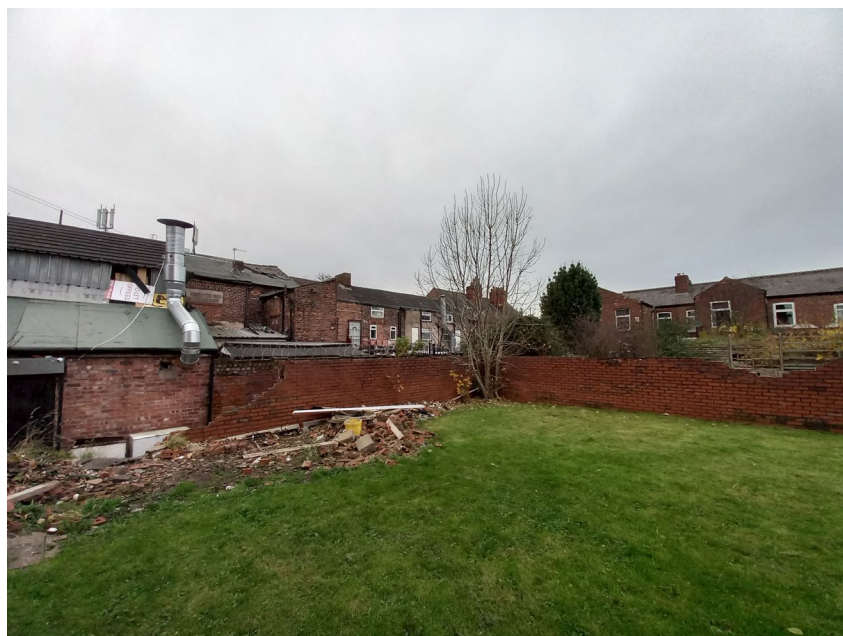
View of the eastern corner of the site showing collapsed boundary wall.
