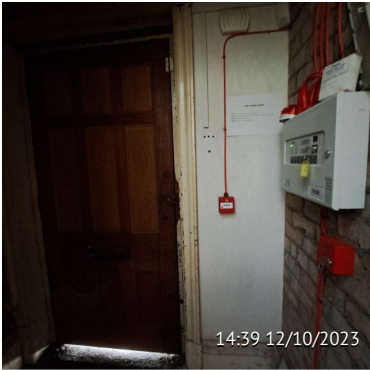
Existing Equipment Existing call point and fire alarm panel
