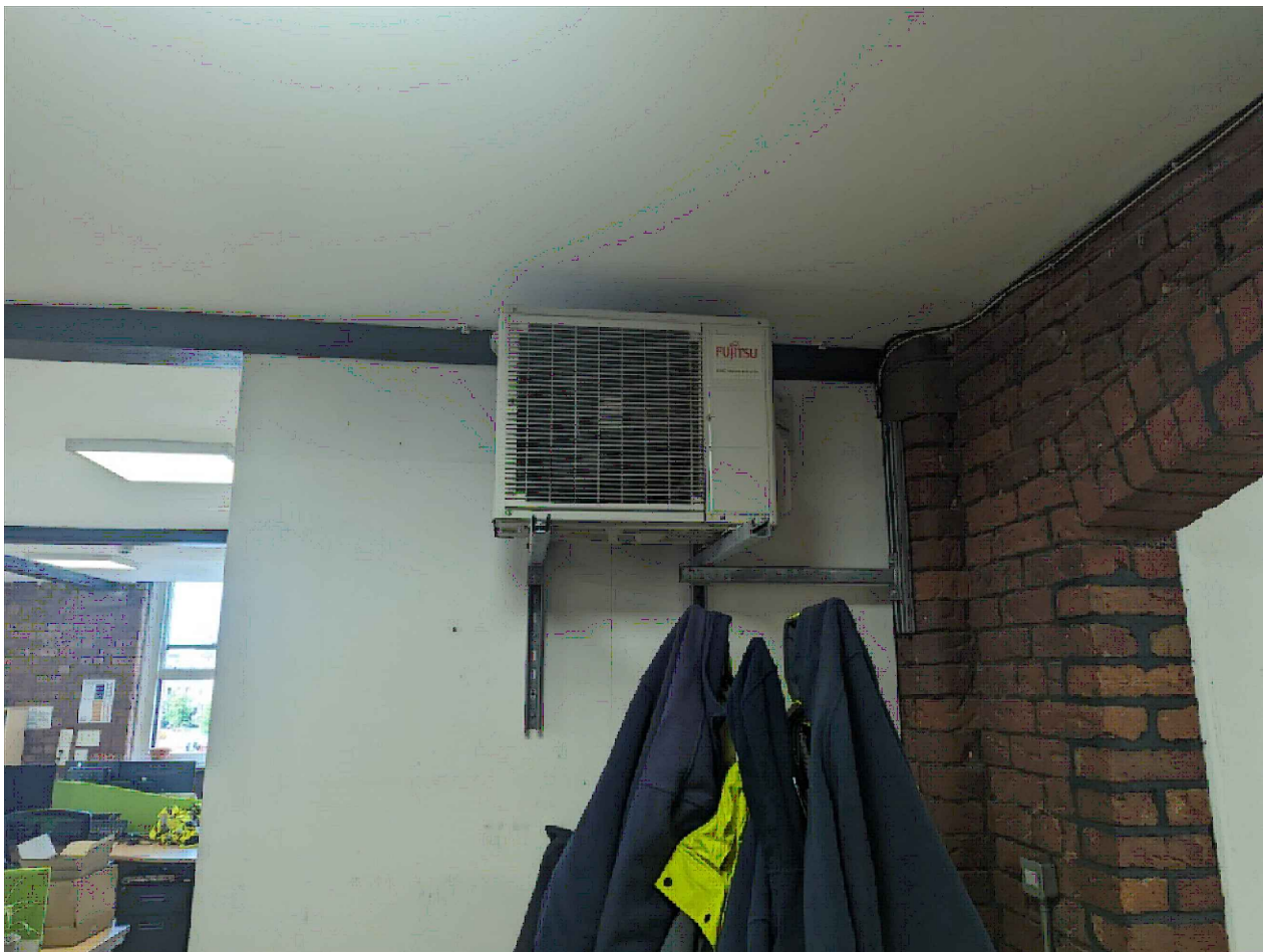
Photo 04 View of the non compliant AC condenser mounted internally serving the Comms Room.
