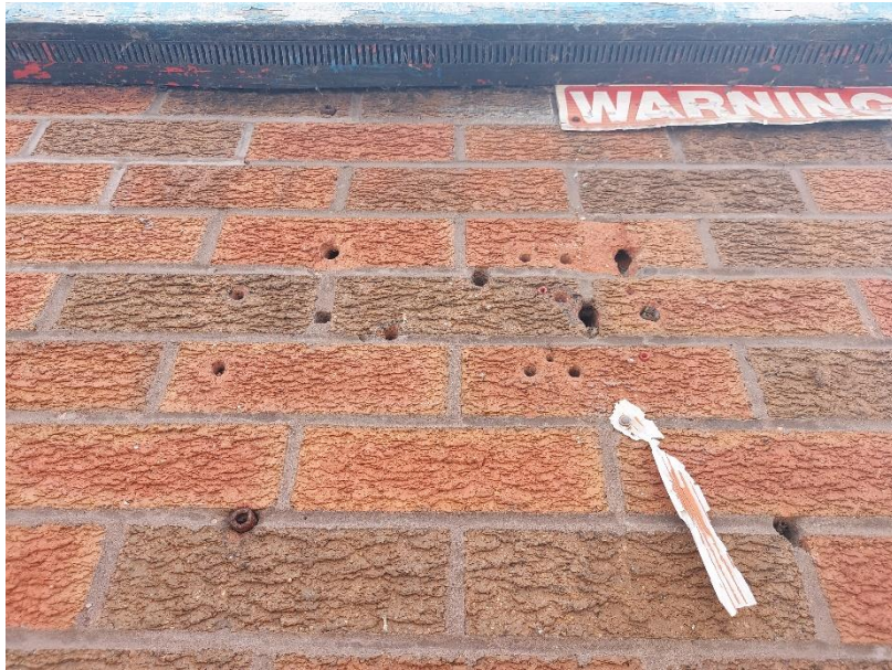
PLATE 5 SHOWING DAMAGED BRICKWORK
