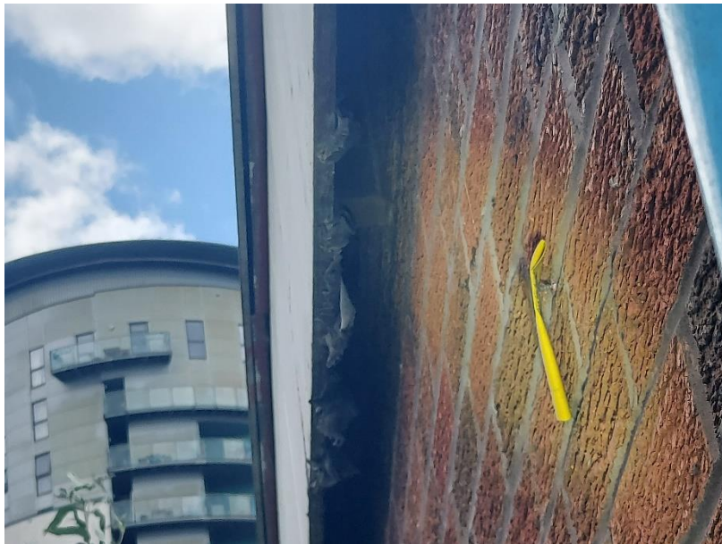
PLATE 6 SHOWING GAP UNDER FASCIA
