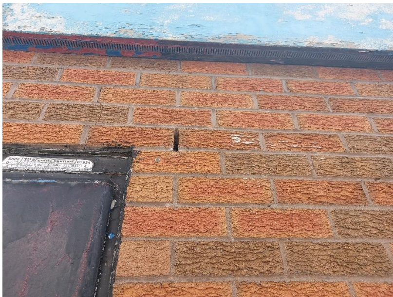
PLATE 4 SHOWING WEEP HOLE ON NORTH-EAST FACING ASPECT
