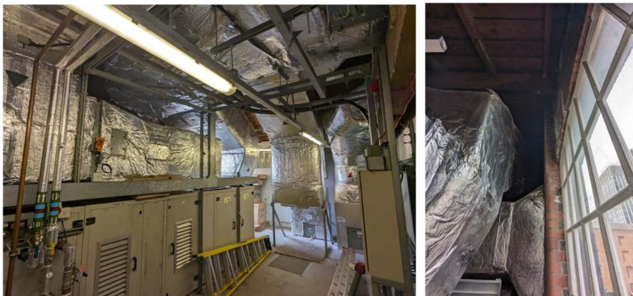
Figure 3-1 Examples of heavily congested spaces along northern edge of New Warehouse, limiting strengthening options
