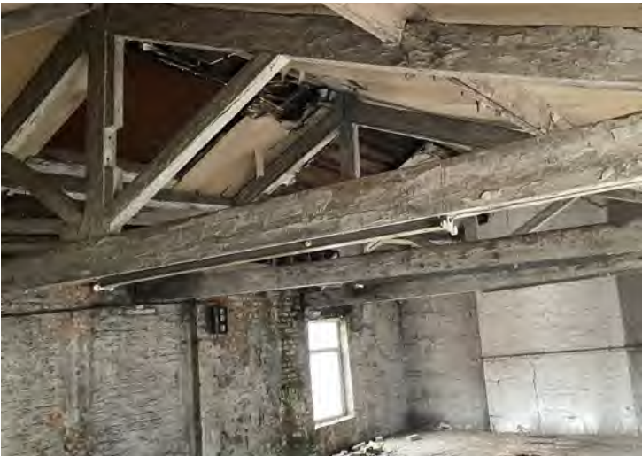
Fig. 69 Condition of No 56-58 Lever Street
