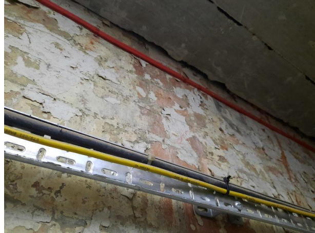
Plate 15: Building B5 Crevice Feature at Internal Wall Top
