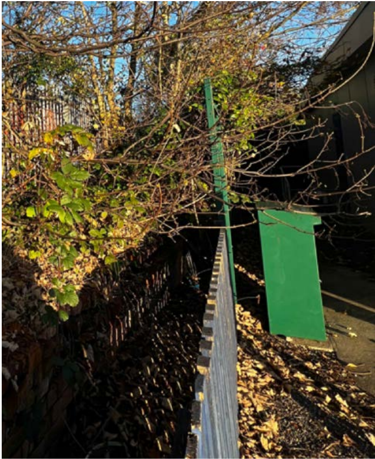
EXISTING RIGHT OF WAY - OVERGROWN
