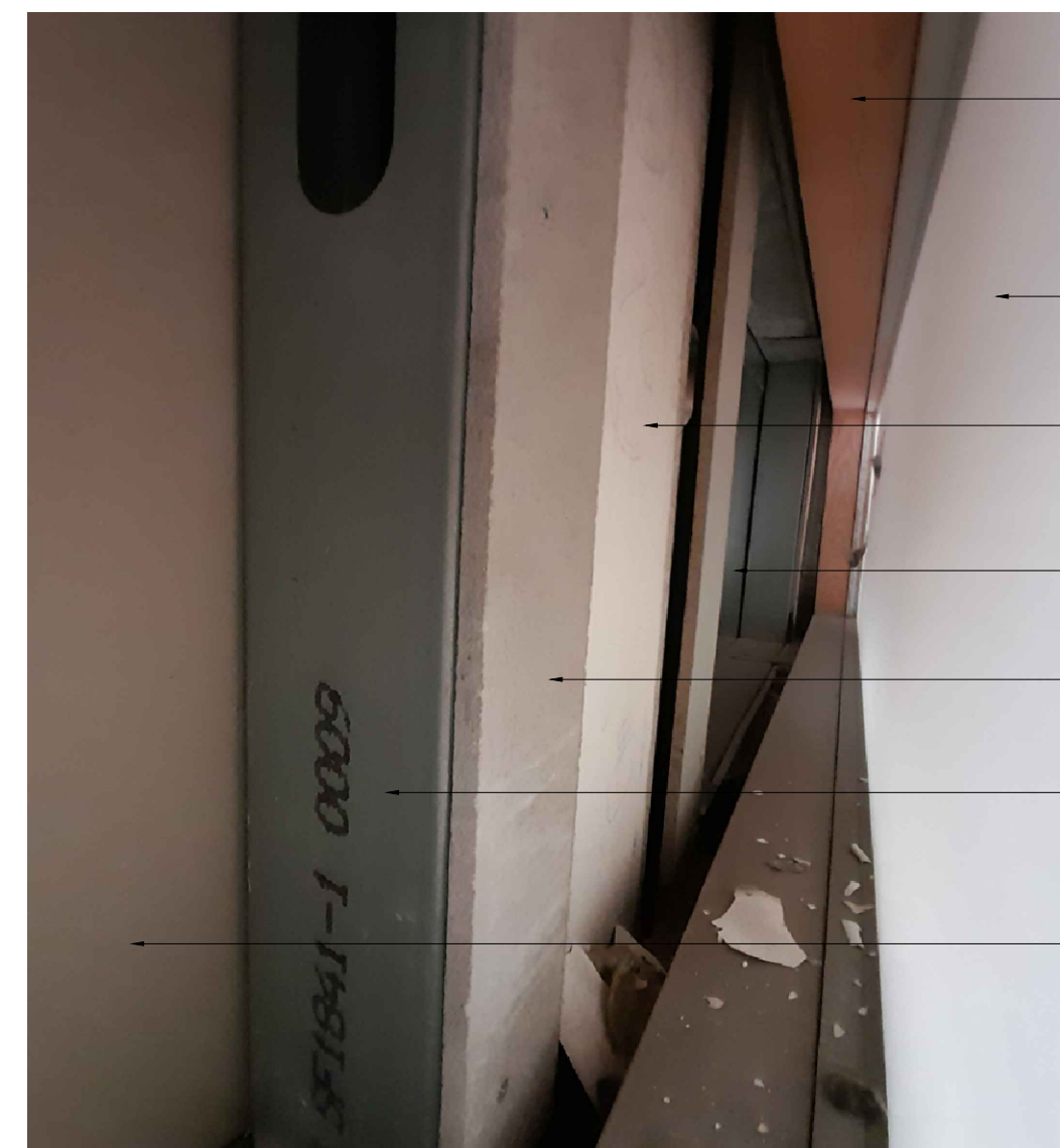
PICTURE 03 - OPENING UP BEHIND STRIP WINDOW LEVEL 5 NOTE: NO VERTICAL CAVITY FIRE BARRIER BETWEEN BACK OF WINDOW AND FACE OF COLUMN. NOTE COMPARTMENT WALL STOPS AT COLUMN.
