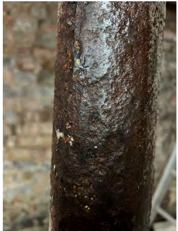
Fig.19 wiping down column 2 reveals rust and no paint.
