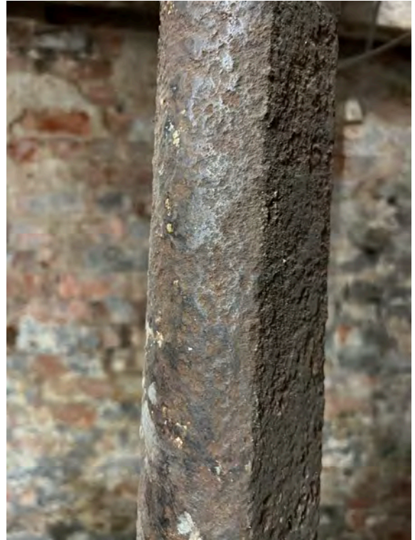
Fig. 21 column 3 is majority rust covered but there are small areas of black paint.
