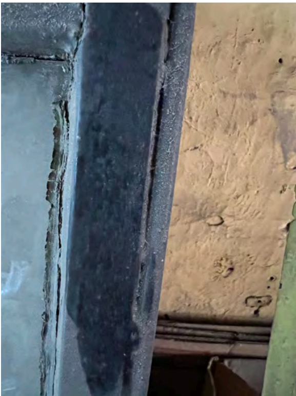
Fig.7 External side of second floor front window, top layer of black gloss paint
