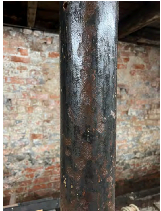
Fig. 17 Column 1 showing visible black paint.
