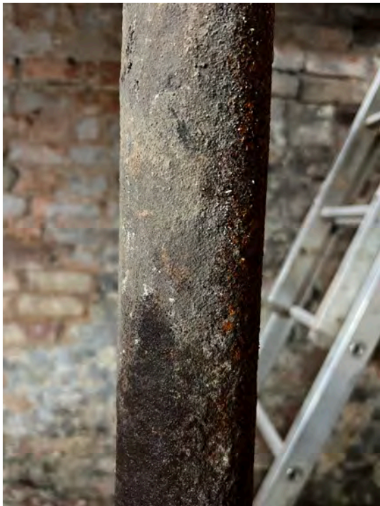
Fig.18 column 2, dirt and rust present.
