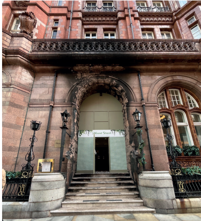
Fire damaged West Entrance - current condition
