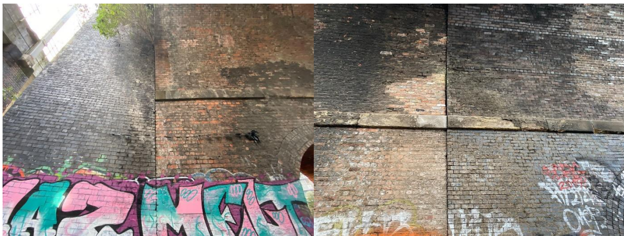
Figure 1: Gaps between the Network Rail arches and southern abutment
