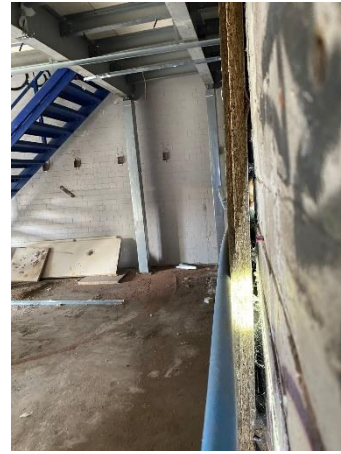
Figure 4: Gap between plywood and brick wall.
