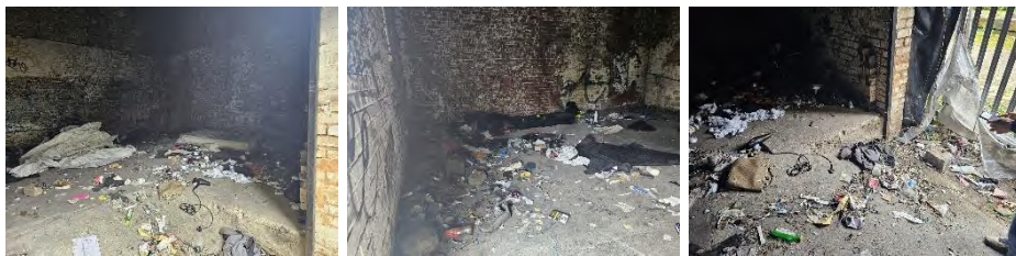
Images inside of cold store 2.
