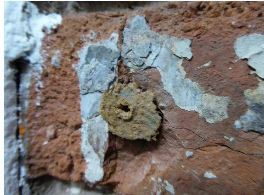
Figure 20: evidence of historic blue-grey decoration surviving to the lower ground floor.
