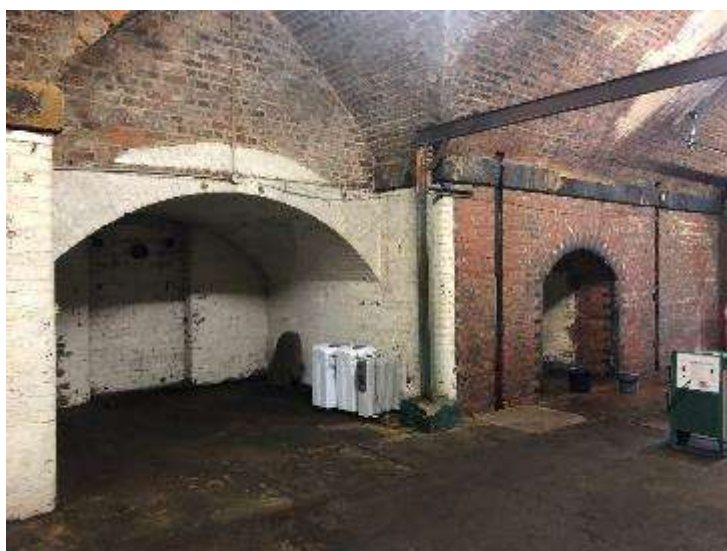
Figure 28: Blocked arched underpass, previously would have permitted access from the undercroft onto Great Bridgewater Street. The blocked doorway dilutes the historical and evidential value of the original plan form. To reinstate this as an active entrance would re-establish this value. The recessed arch featuring the former entrance is of considerable significance and to reinstate it would be highly recommended.
