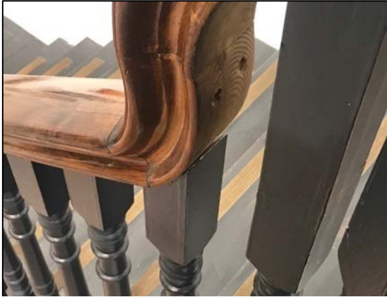
25. Detail of staircase showing modern timber balusters loosely fitted to finely detailed original carved hardwood handrail.
