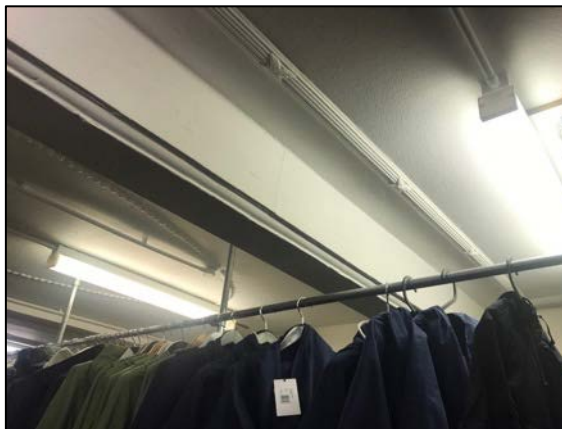
7. Anomalous decorative chamfer to enclosed structural beam within basement.
