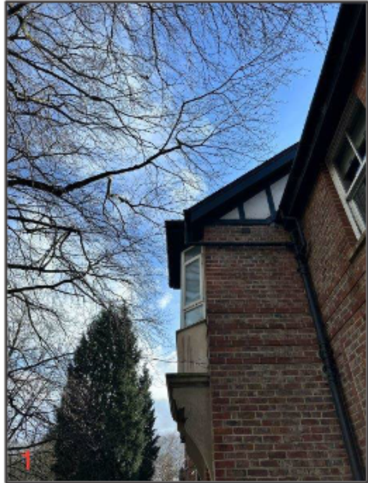
Picture 3. T1-Branches touching building.
