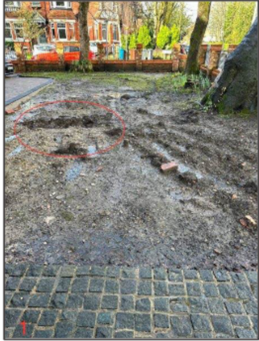
Picture 1. T1-Beech located at front of the house. Excavation and root severance evident (red ellipse).
