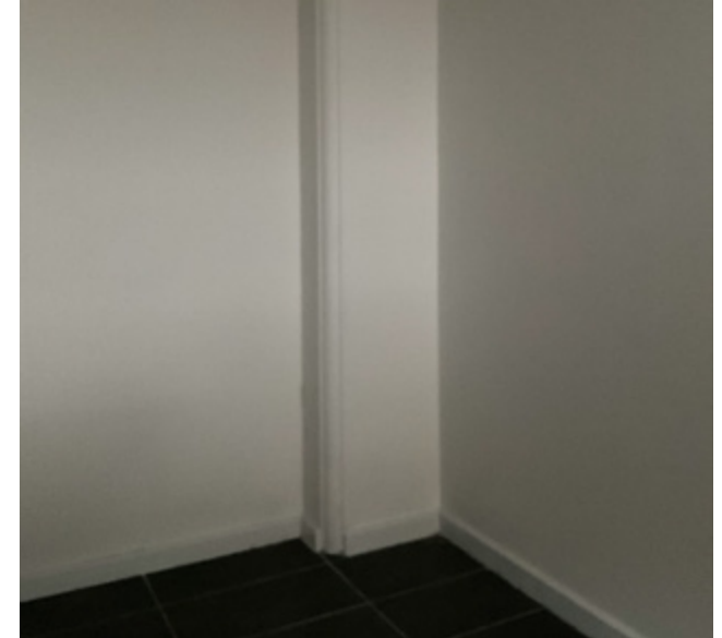
3.81 No. 23, plain replica moulded edge to the former lightwell opening
