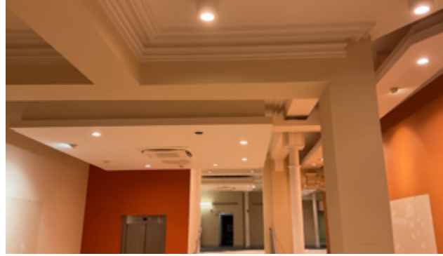
3.32 No. 17, nubbin and column preserving line of the inner wall of the lightwell
