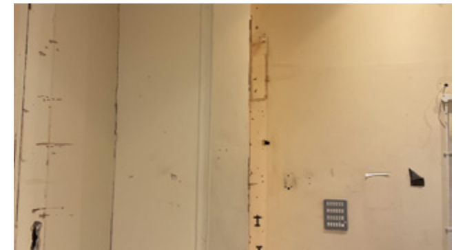
3.45 No. 19, west wall (L) and lightwell opening with bracket, the west wall to the lightwell lost
