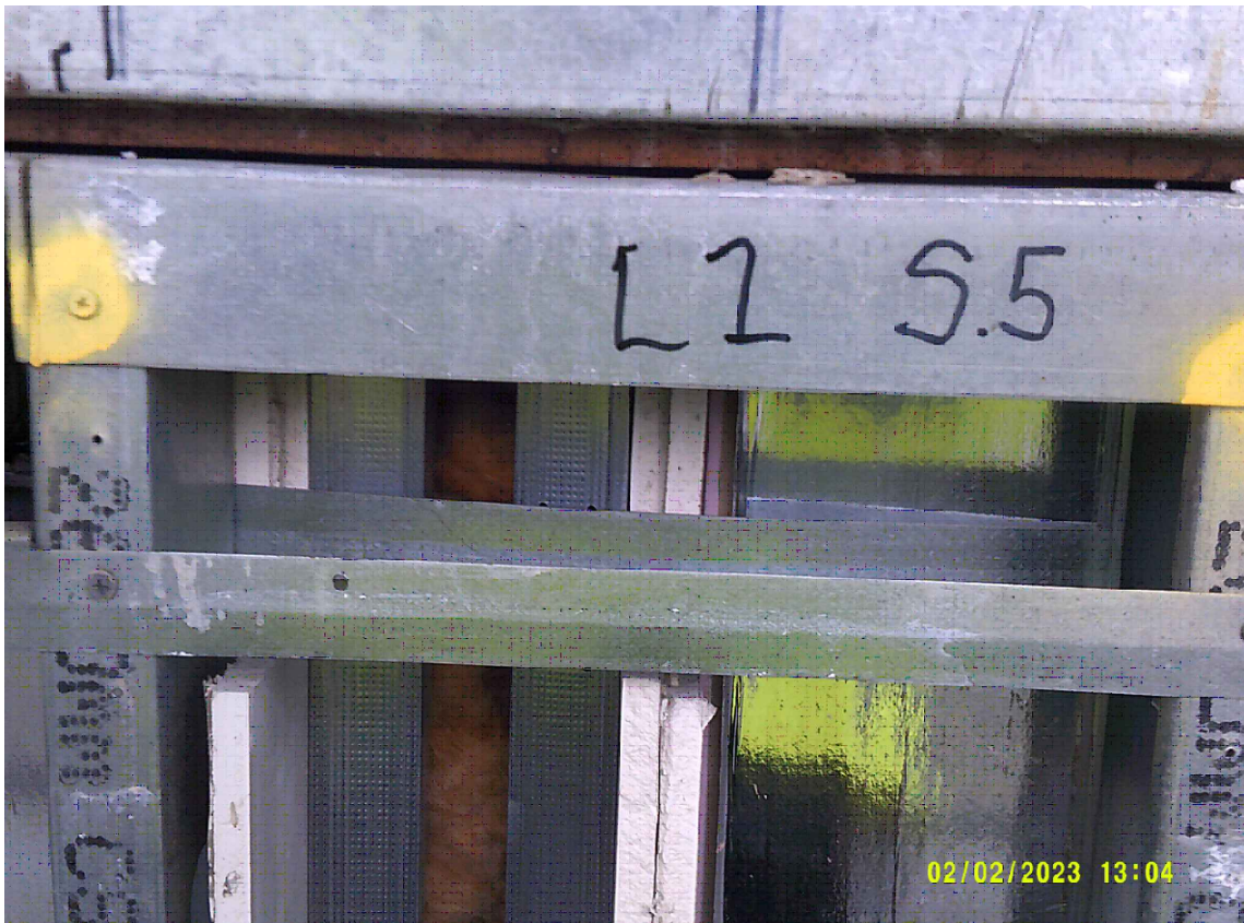
EXAMPLE OF EXISTING METAL FRAMING BREACHING COMPARTMENT WALL. TO BE CAREFULLY CUT OUT AND REMOVED TO S.ENG ADVICE.
