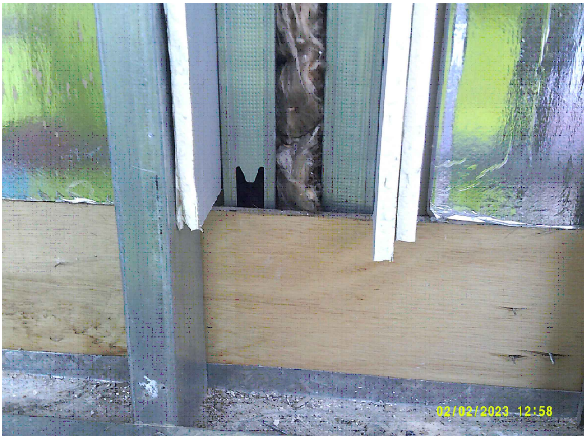
EXAMPLE OF EXISTING SKIRTINGS BREACHING COMPARTMENT WALL. TO BE CAREFULLY CUT OUT AND REMOVED.
