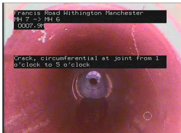
MH 7X_89b47a5e-344b-4ec8-8955-deaf61bfc5f2_20210826_1225 02_691.jpg, 00:01:17, 7.90 m Crack, circumferential at joint from 1 o'clock to 5 o'clock
