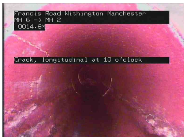
MH 6X_00ad8361-1e3f-4166-ae31-f61304383bb2_20210826_123 501_064.jpg, 00:02:47, 14.60 m Crack, longitudinal at 10 o'clock
