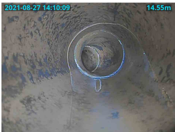
Branch AX_0926991d-9f18-47d7-b176-fb91759953fe_20210901_150 130_870.jpg, 00:00:48, 14.55 m Crack, circumferential from 12 o'clock to 12 o'clock
