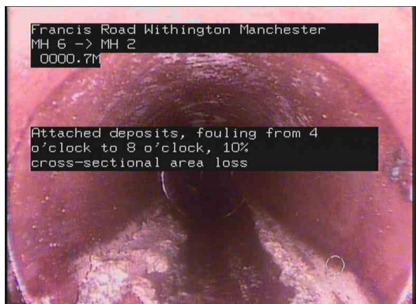
MH 6X_baf85516-2245-4ef0-a9f2-7859f030d3a3_20210826_123152_565.jpg, 00:00:21, 0.70 m Attached deposits, fouling from 4 o'clock to 8 o'clock, 10% cross-sectional area loss
