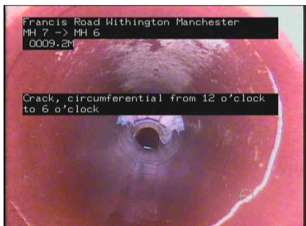
MH 7X_c9e9c15c-2a03-4162-b3da-067901e5d981_20210826_12 2523_300.jpg, 00:01:31, 9.20 m Crack, circumferential from 12 o'clock to 6 o'clock
