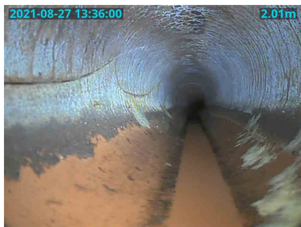
Branch AX_6146da81-8ca1-470e-ad6c-73b35c180b2b_20210901_15 4734_671.jpg, 00:00:16, 2.00 m Crack, longitudinal at 9 o'clock, start
