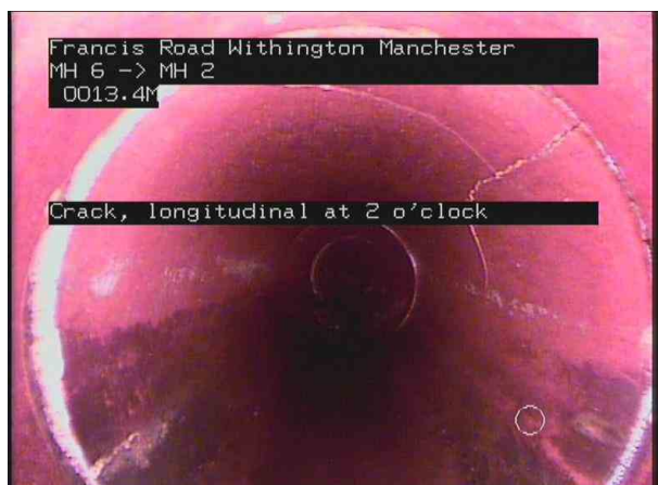
MH 6X_ff37d770-b7c1-479b-9ce7-76d537fff7b8_20210826_12344 4_706.jpg, 00:02:33, 13.40 m Crack, longitudinal at 2 o'clock
