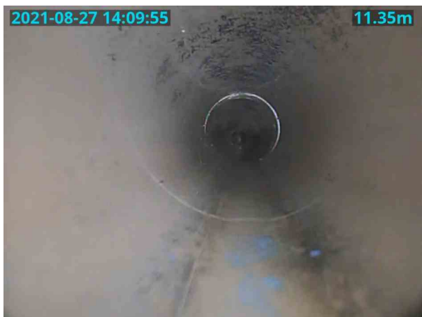
Branch AX_fa7d7cbc-cd8b-4926-82d2-457244cd1665_20210901_150 029_987.jpg, 00:00:34, 11.35 m Crack, circumferential from 12 o'clock to 12 o'clock
