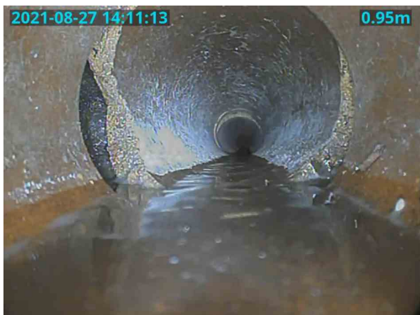
MH 8X_a92836fb-08e2-4164-8299-4596a40a9081_20210901_145602_292.jpg, 00:00:10, 0.95 m Broken pipe at joint from 6 o'clock to 9 o'clock
