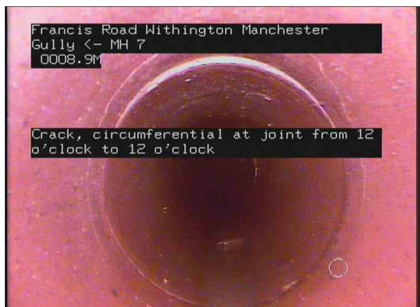
GullyX_536c09ae-1472-4357-b9f2-305f556a547e_20210826_122022_207.jpg, 00:01:24, 8.90 m Crack, circumferential at joint from 12 o'clock to 12 o'clock
