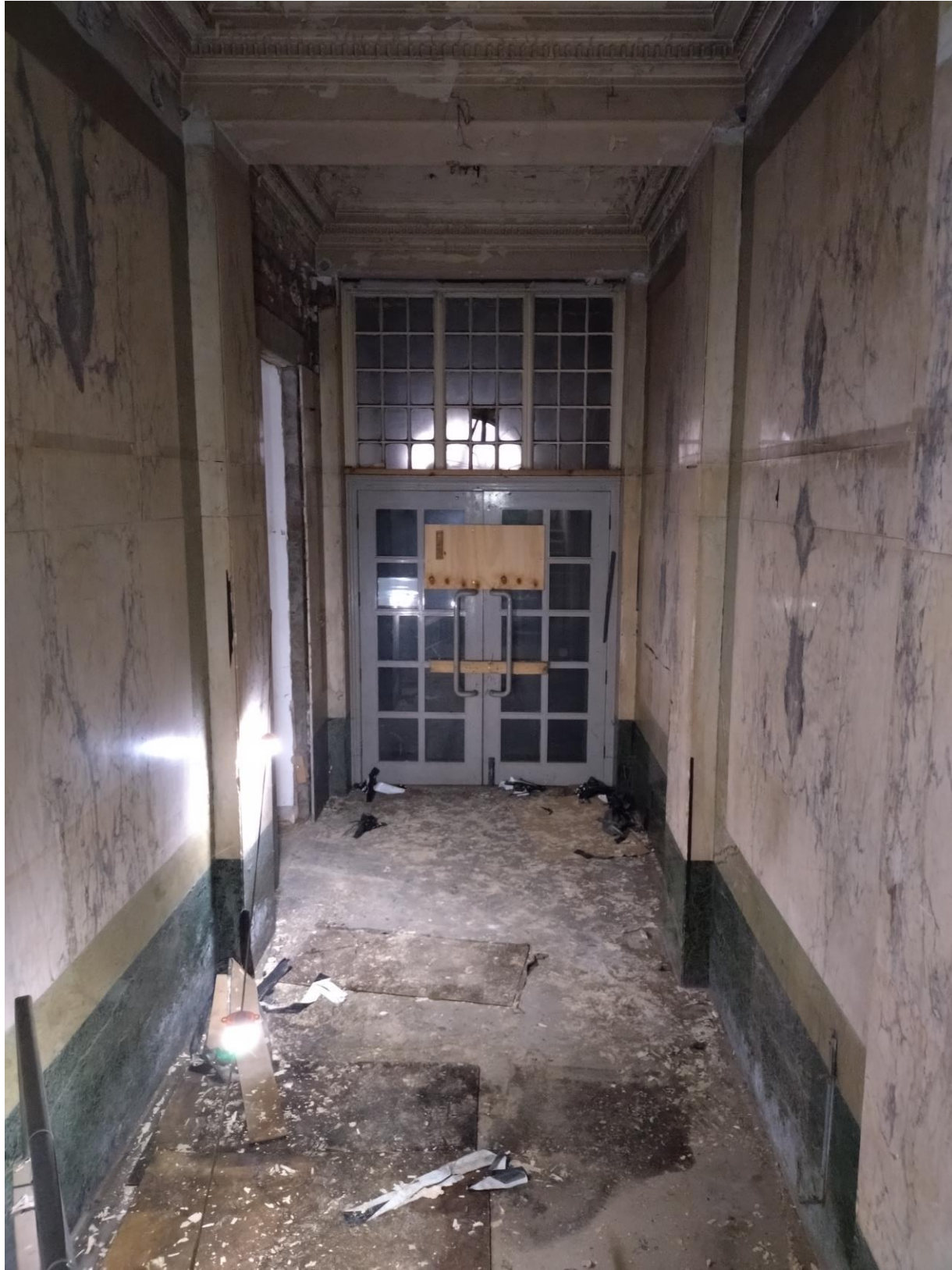
Current condition with entrance obstructed and general state of dis-repair
