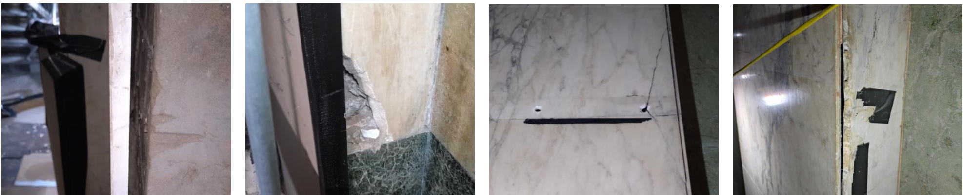
Photos documenting the thin material thickness and general damage to significant portions of the marble from past interventions
