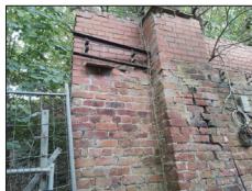
U2 - No brick work to left of image, fence to be replaced as Hydrock recommendation.
