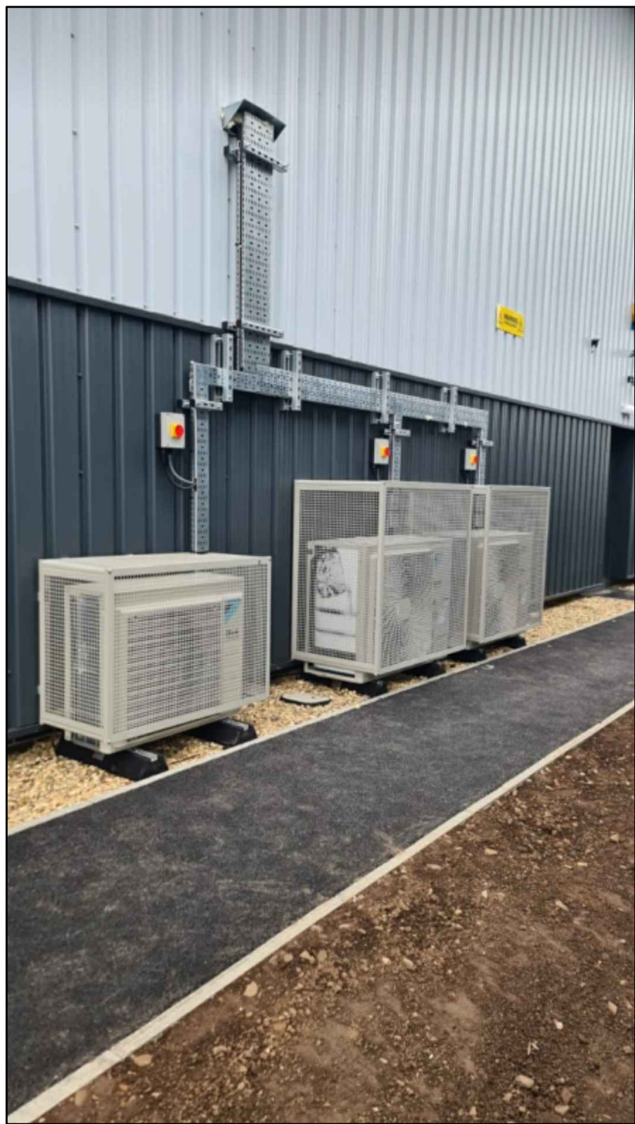
PHOTO OF TYPICAL ASHP CONDENSER UNITS & SECURE CAGES NOT TO SCALE
