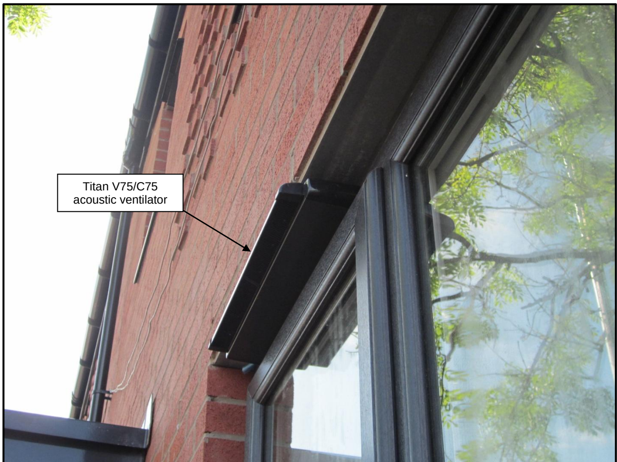
Photograph 6. Titan V75/C75 acoustic ventilator, plot 10 - front elevation
