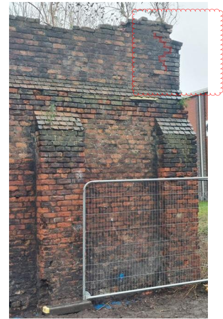
Panel 10: Wall Defect / Deterioration Checklist
