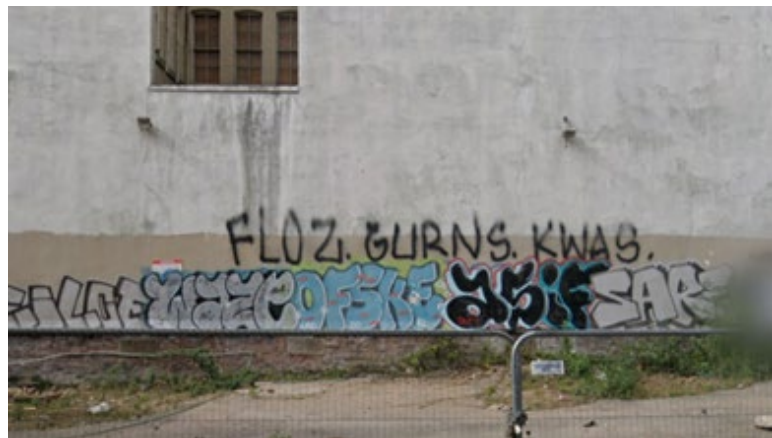
Figure 2: Google Street view image showing graffiti and mis-matched paint on the exterior wall of 12 Piccadilly (April 2021)
