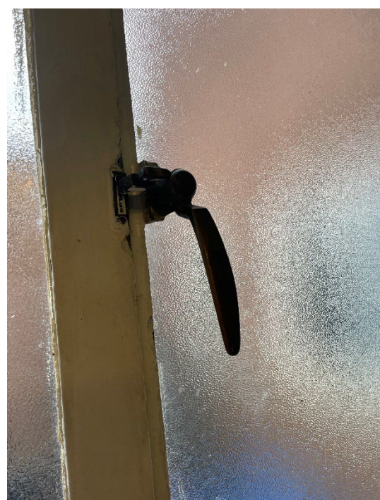
Figure 69: Changing room 2.2, north-east corner. Original 1950s brass window latch detail.
