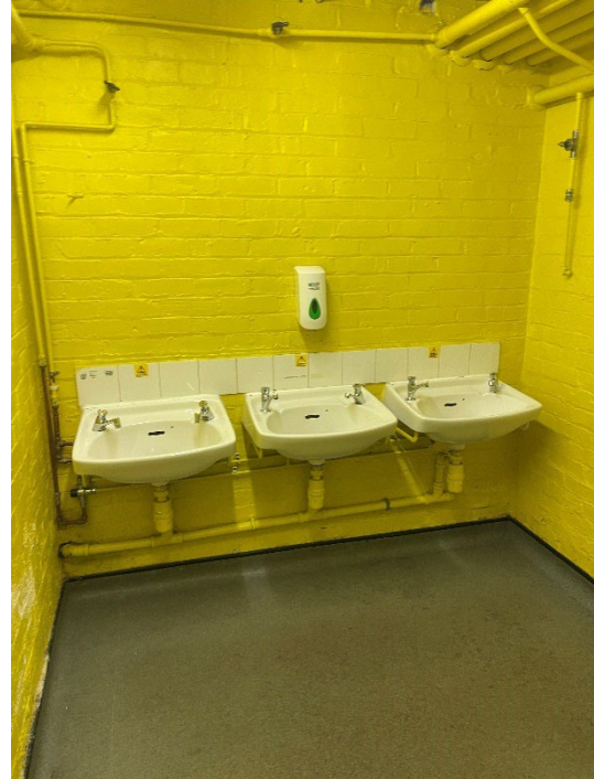
Figure 94: Fixed sinks. East wall to NW toilet room.
