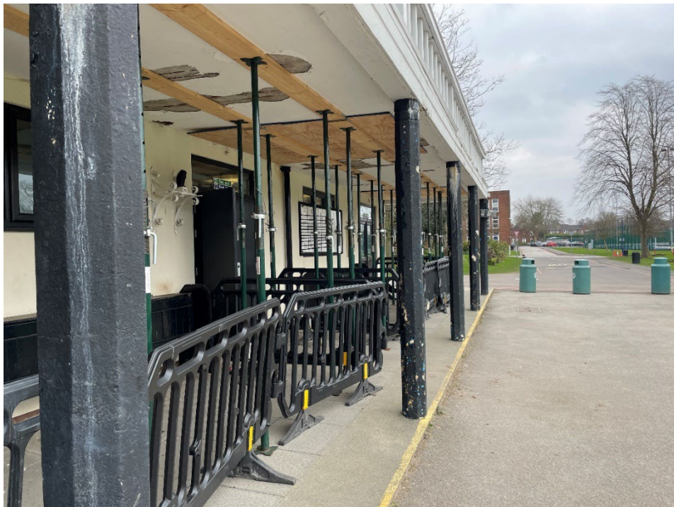
Figure 18: View of the south elevation, looking east across veranda. Currently propped with temporary supports. Six original columns feature. Blue paint visible below black coating.
