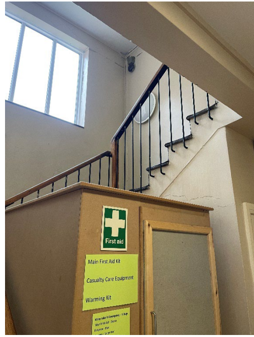
Figure 103: Original 1950s baulustrate detail.
