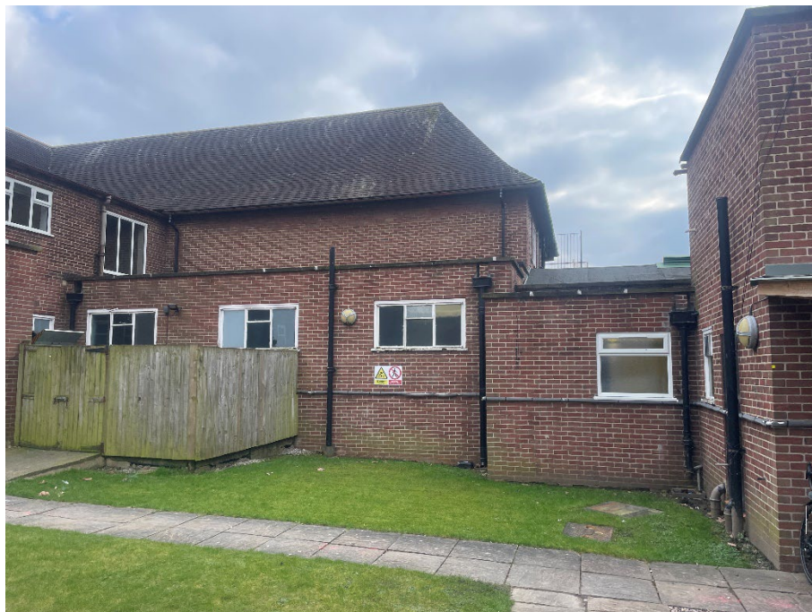
Figure 31: View of the north elevation of the pavilion (centre). Note modern, replacement windows and doors. Original rainwater goods, later timber enclosure.
