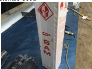
Evidence of Juta GPSAM
