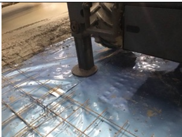
Plant keeping off the mesh on the membrane
