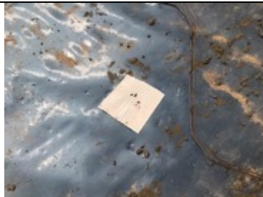
Defect sealed using SAGM and heat applied
