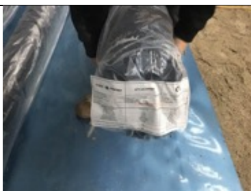
Evidence of Juta GP5 gas membrane
