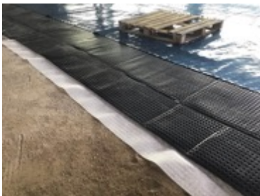
Vent mat installed under the mezzanine floor area
