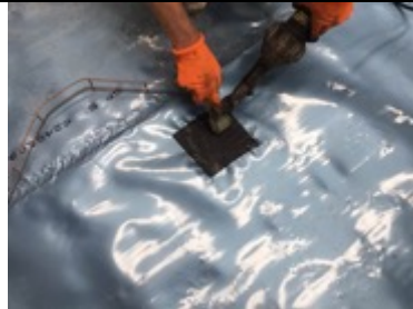
Recorded defect sealed using SAGM and heat applied
